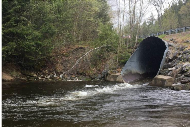
The existing culvert constricts the stream at the outlet.
