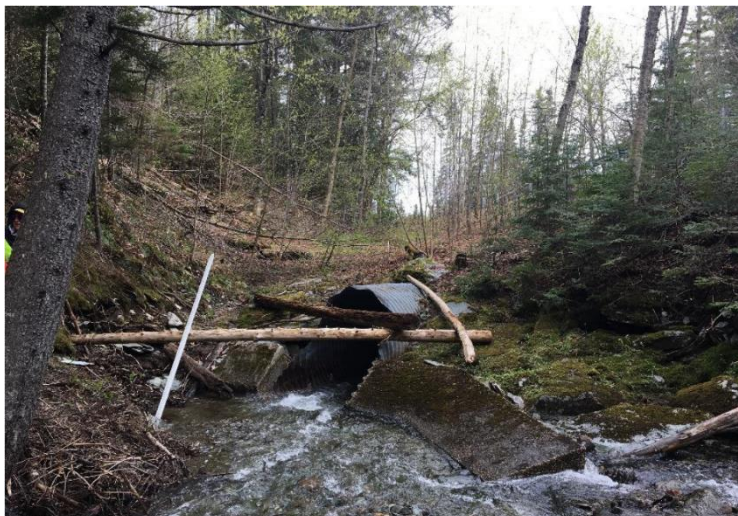
An undersized culvert and an inadequate alignment will cause debris build up at the inlet
