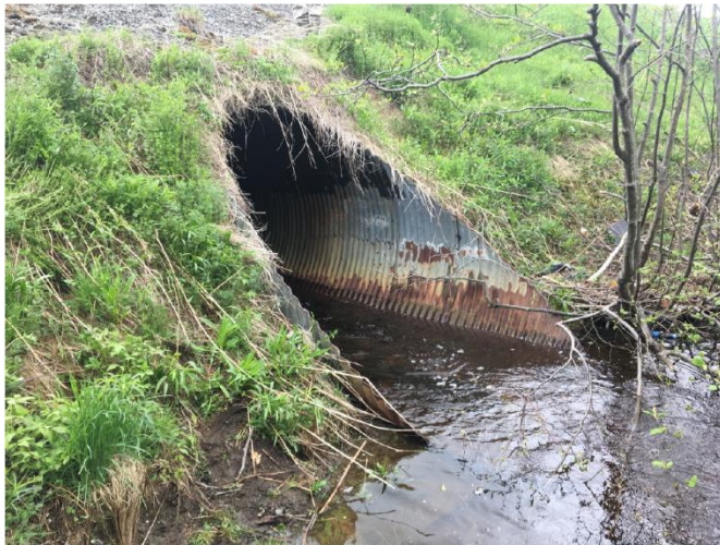
A constricting existing culvert will be replaced with a 4-sided concrete box that meets the ANR bank full width.
