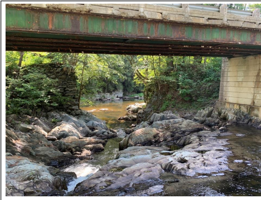
Upstream of structure looking downstream. Cracks in abutment may provide bat roosting. September 10, 2019
