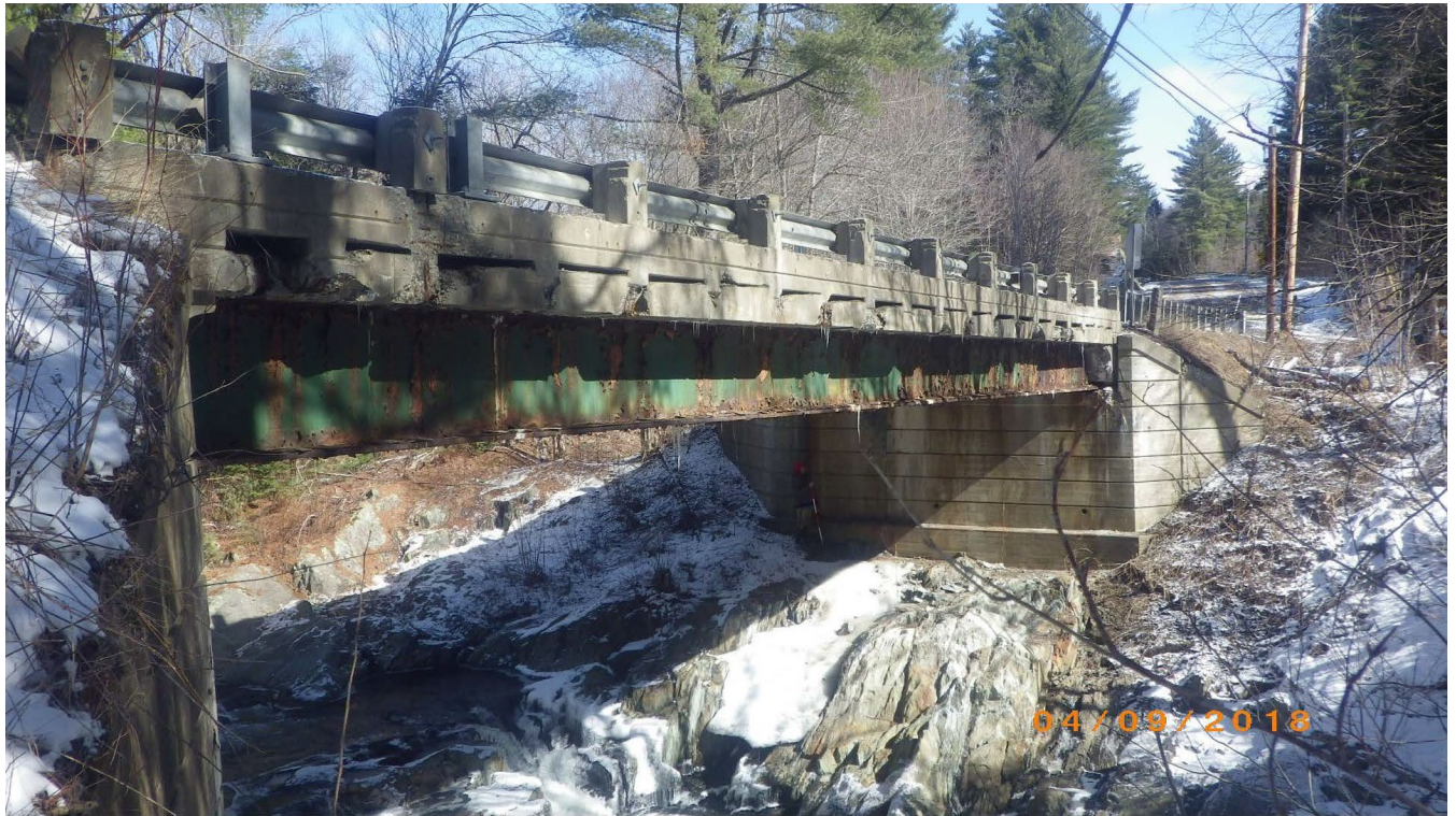
Figure 3: Note the bridges original Art Deco detailing and poor substructure.
