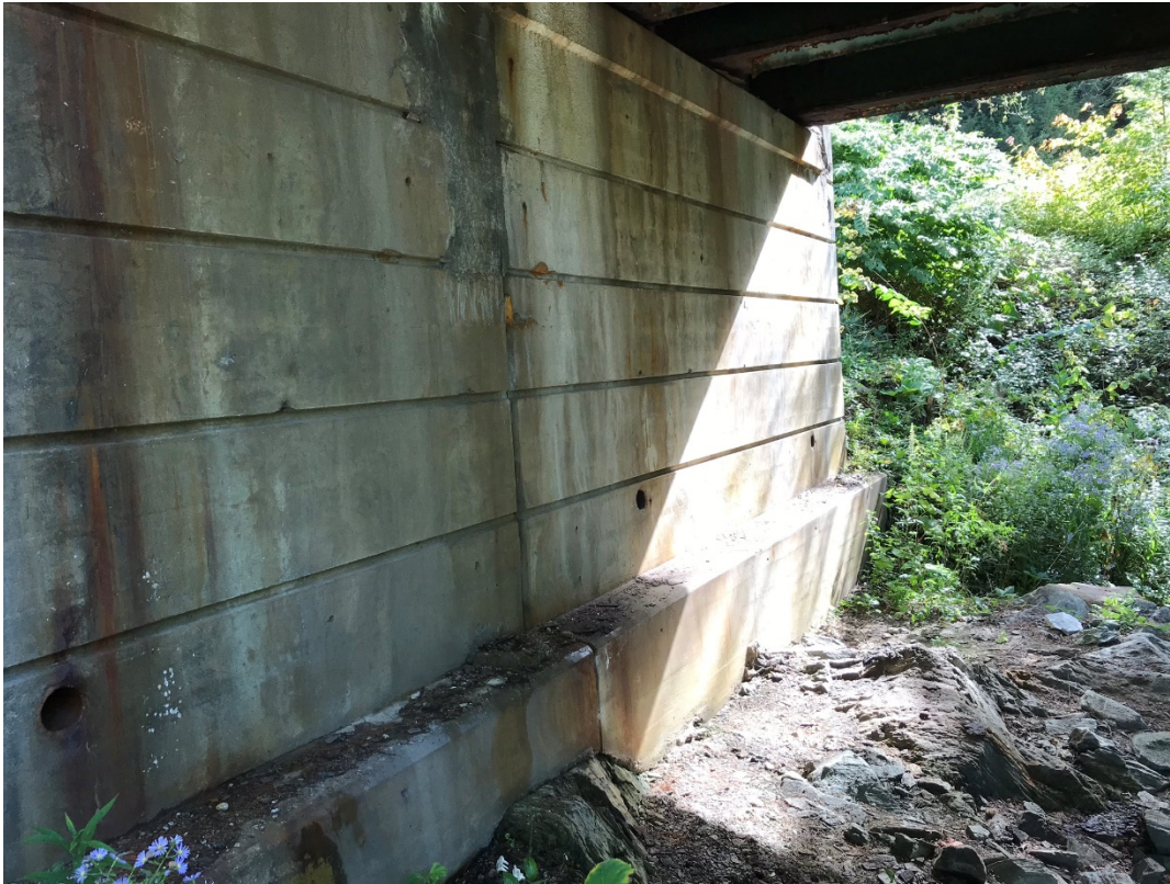
Figure 3.6: Facing northern abutment outlet; note exposed bedrock at bottom of footing elevation for abutment.
