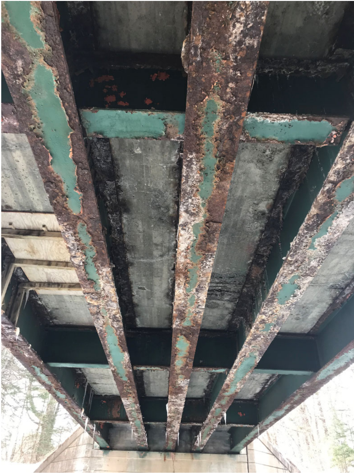
Photo 7: Spalling in deck (Note deck repairs and paint failure at beams)
