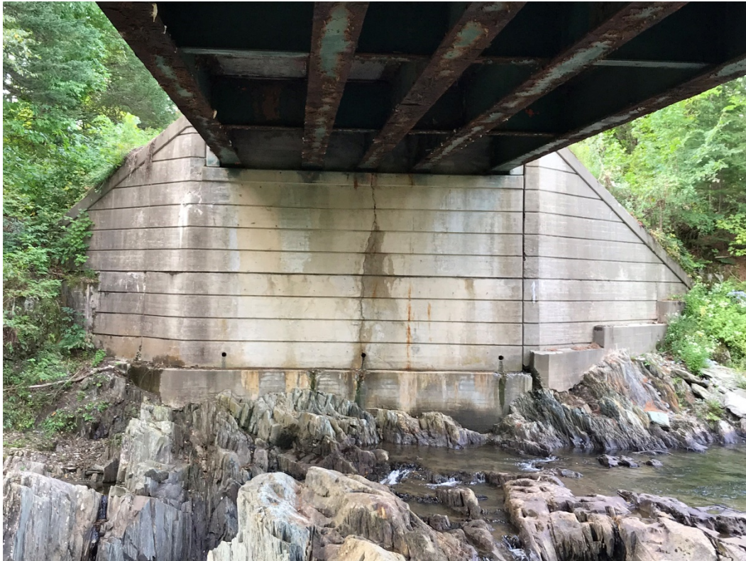
Figure 3.4: Facing southern abutment; note exposed bedrock at bottom of footing elevations for abutment and wingwalls.
