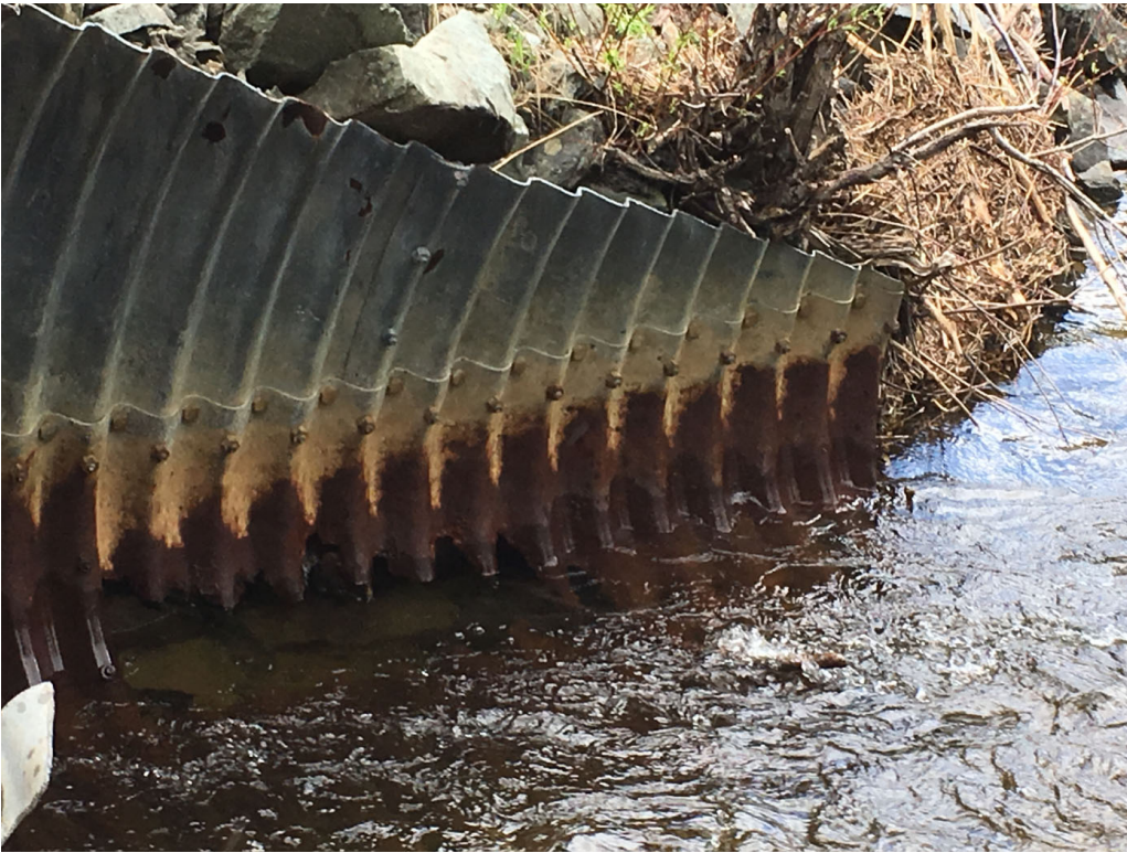
Picture 6: Hole at Outlet Waterline
