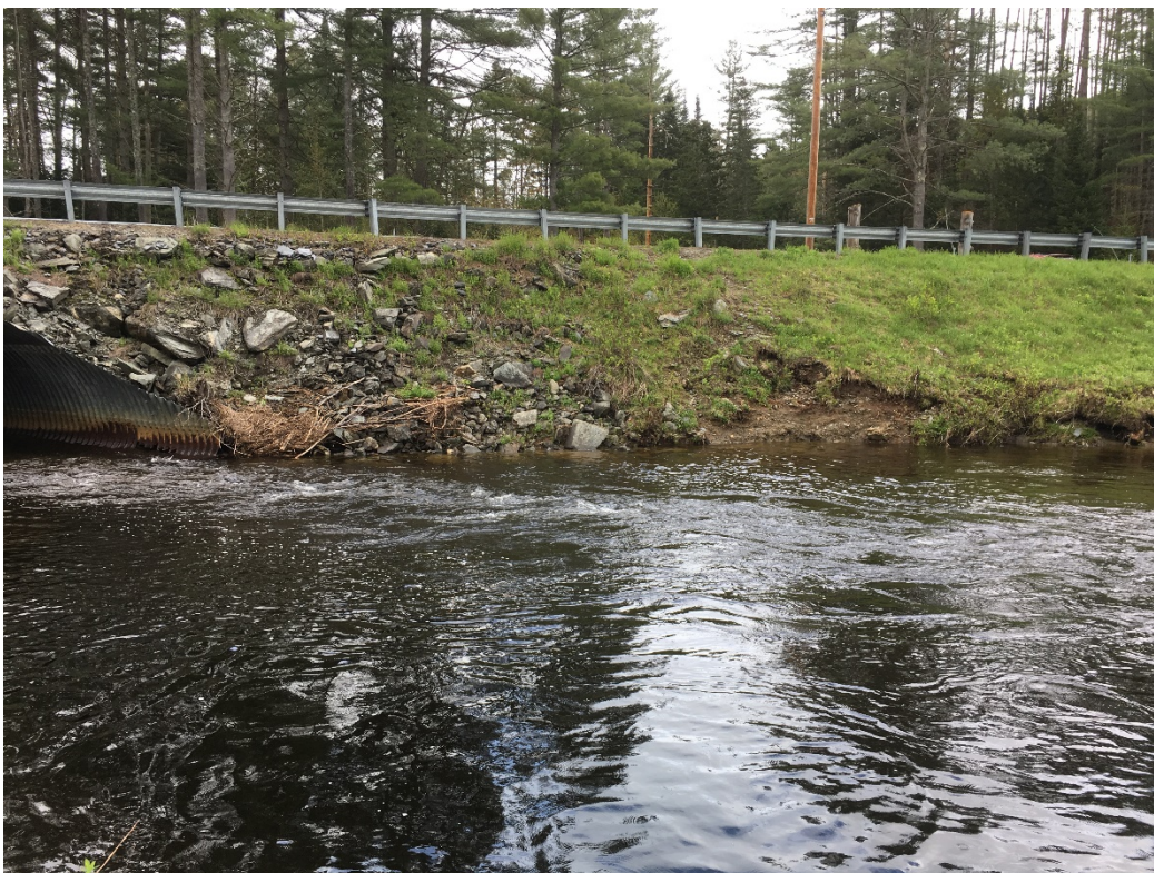
Figure 3.2: Sloughing of slope near the outlet. [Structures photo dated May 2019]
