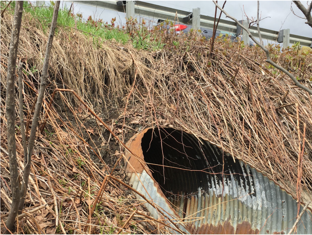
Picture 7: Scour Hole Above Bridge 94
