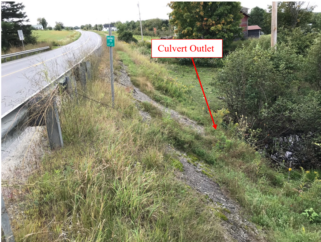
Figure 3.3: Facing culvert outlet; note sloping embankment that may preclude drilling from directly adjacent to culvert outlet.
