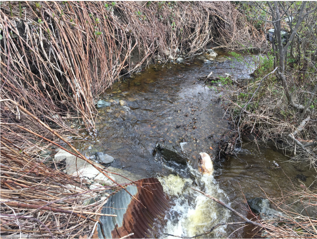
Picture 8: Scour Along Banks
