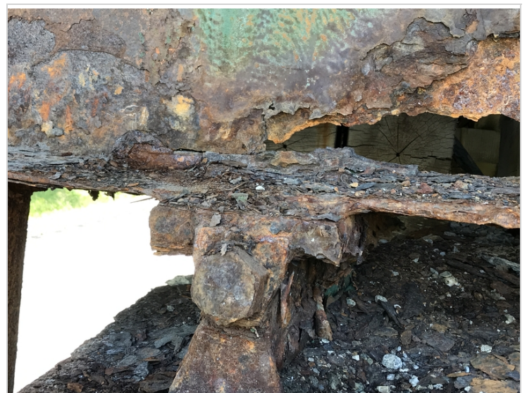
Pier #2 Beam #1 Section Loss
