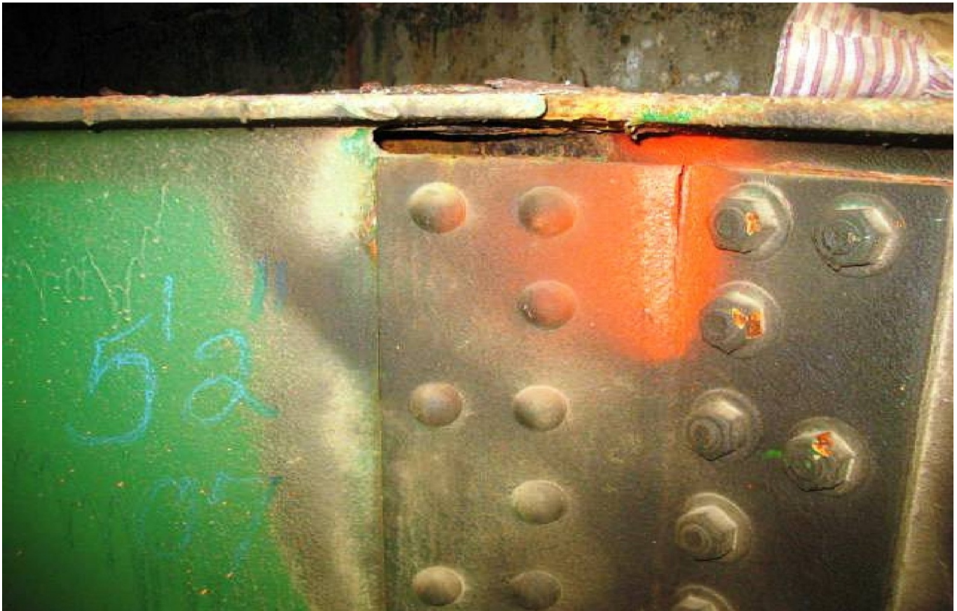
Secondary Member Crack
