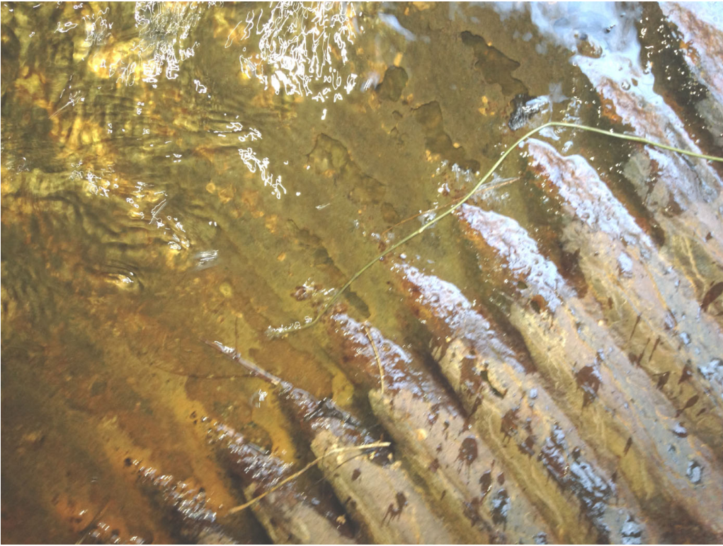
Picture 6: Perforations in Culvert Invert
