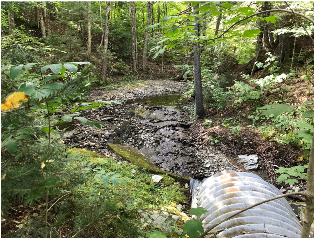
Figure 3.1: Facing upstream; note high frequency of gravel, cobbles, and boulders within streambed and possible bedrock outcroppings.
