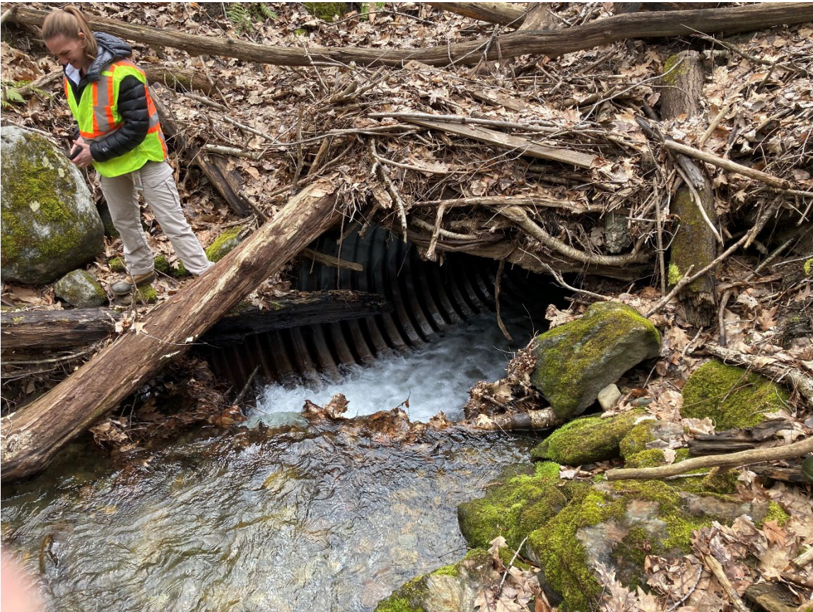
Inlet of PID68002, close up of woody debris.
