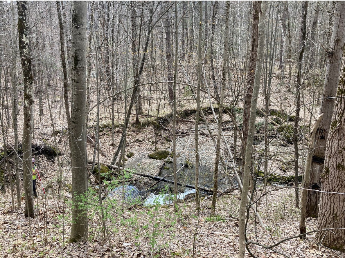
Scour pool view from north of outlet
