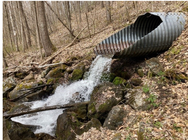
The perched outlet of the existing culvert precludes aquatic organism passage in addition to being detrimental to the passage of mammals
