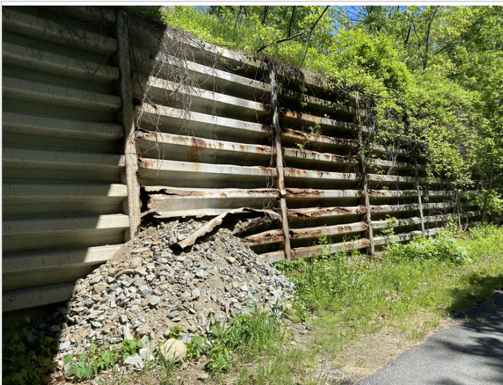
Failing Retaining Wall Northeast Corner
