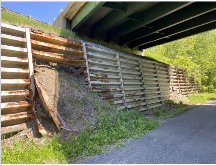
Northern Retaining Wall with Multiple Section Failing
