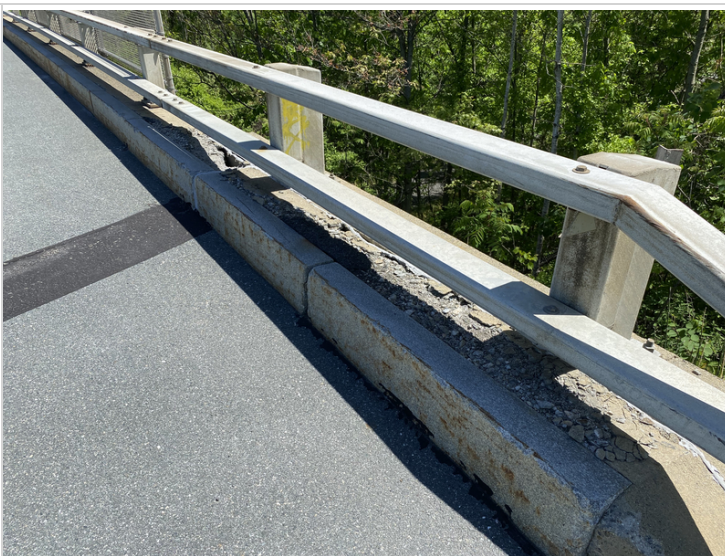
Eastern Curb Spalling / Scaling along the Southern Corner
