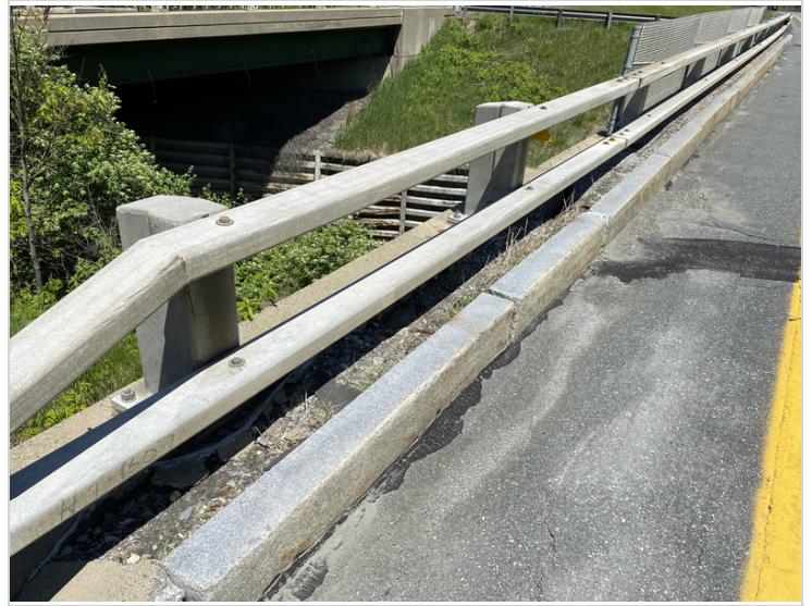
Curb Scaling along Western Side
