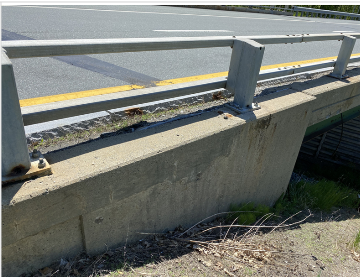
Northwest Curb Scaling / Spalling
