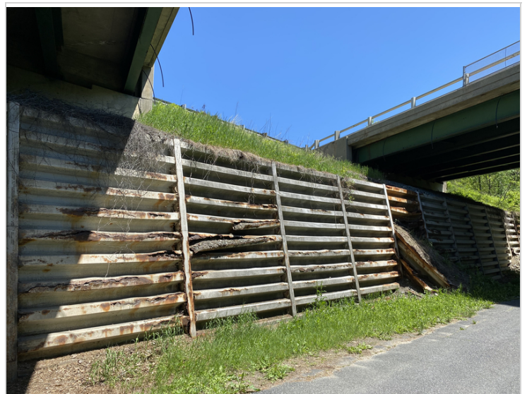
Northern Retaining Wall with Multiple Section Failing
