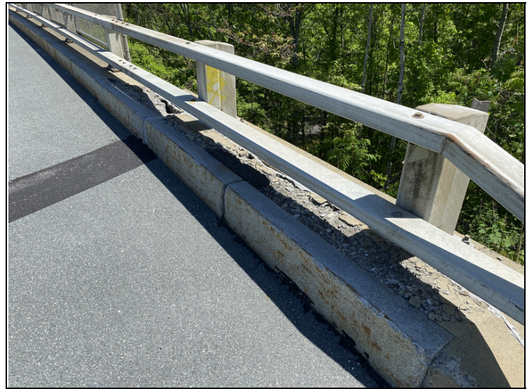
Eastern Curb Spalling / Scaling along the Southern Corner
