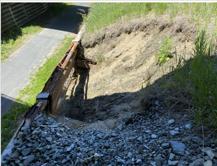
Retaining Wall Blow Out along Northwest Corner of Structure
