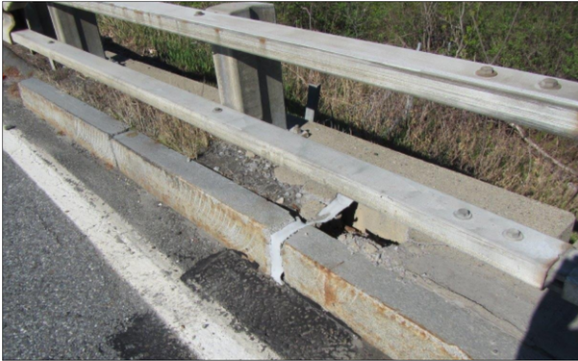
Bridge 27S Curb Deterioration at Bridge End
