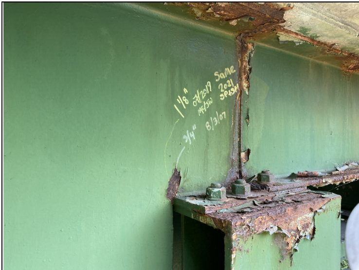
Girder #8 over Floor Beam #1 with ~1-1/8" Crack
