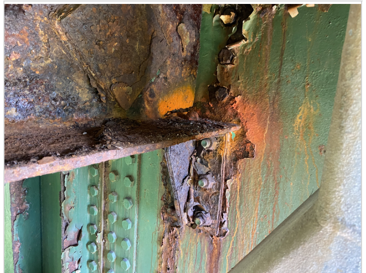
~5-1/2" Perforation along Lower Portion of Web on Beam #7 at Floor Beam #6
