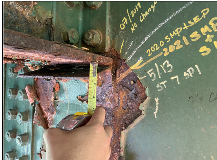
Cracked Weld at Floor Beam #1 West Side along Beam #7 with ~1-1/4" of Downward Transition
