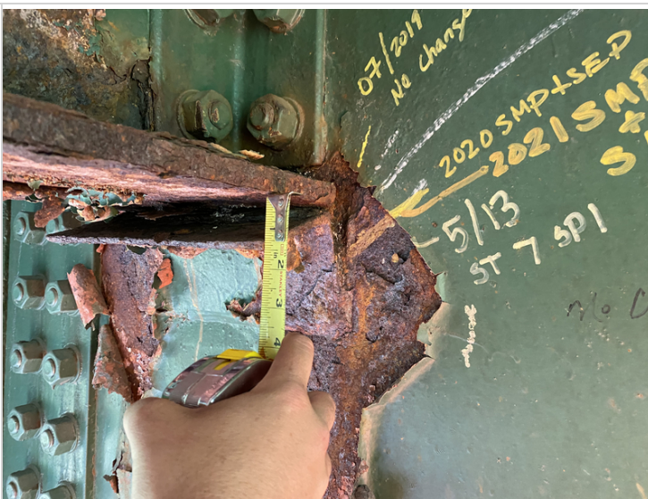
Cracked Weld at Floor Beam #1 West Side along Beam #7 with ~1-1/4" of Downward Transition
