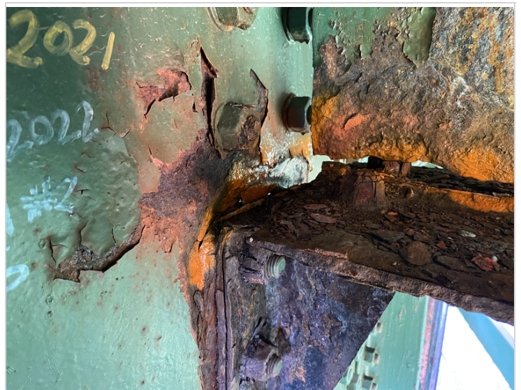
Floor Beam #6 Section Loss at Beam #2 with Perforation
