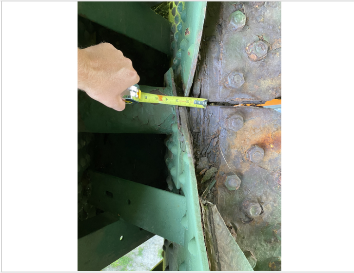
Pack Rust at Upstream Pin at Center of Arch
