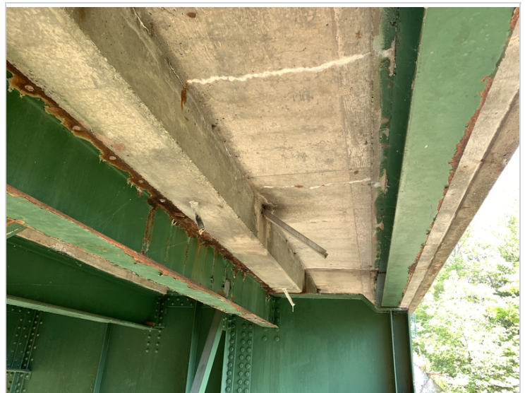
Cracking in Deck in Bay #7 near Abutment #2
