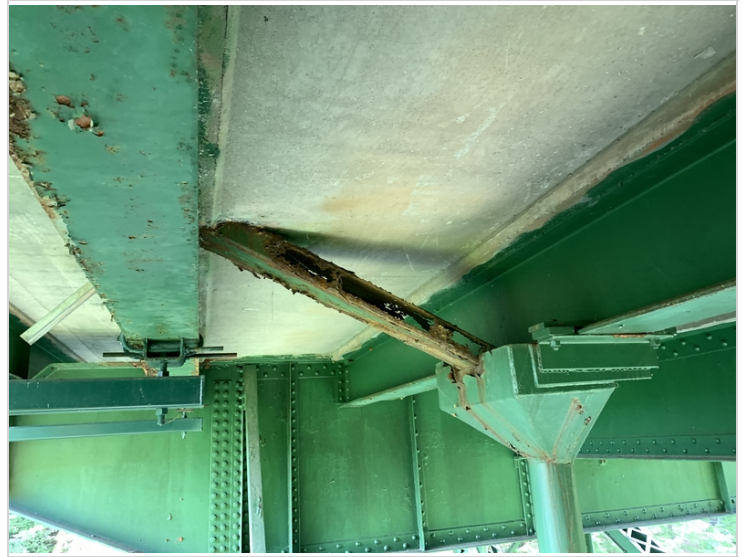
Heavy Section Loss in Deck Drain
