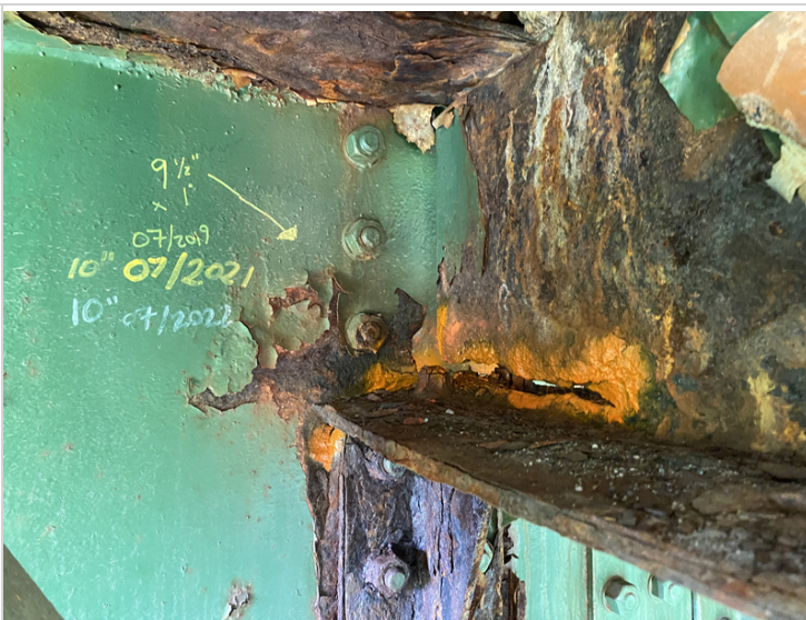
~10" Perforation along Lower Portion of Web at Beam #2 at Floor Beam #6
