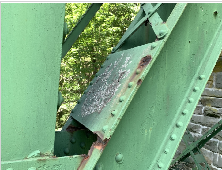
Failed Rivet in Bottom Chord at Diagonal #1 Upstream Side
