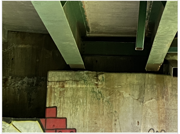
Abutment Cracking below Beam #3
