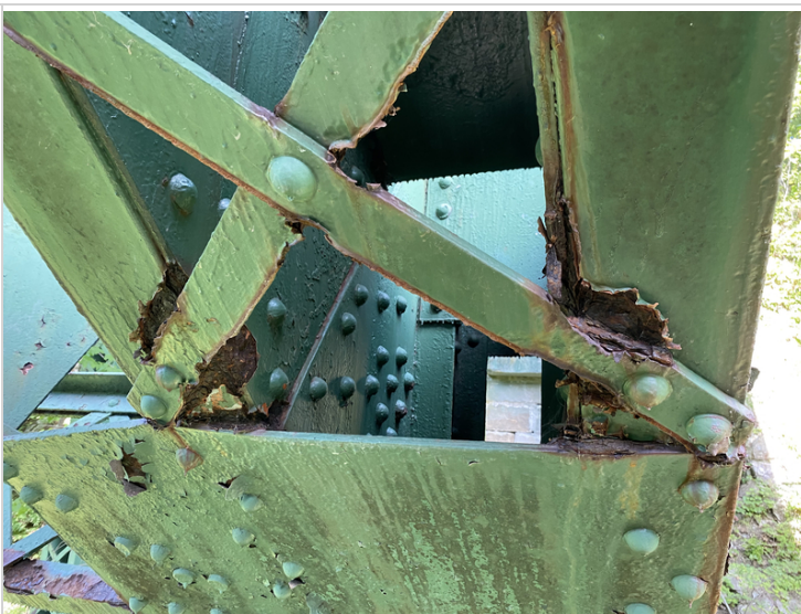
Bottom Chord Section Loss at Vertical #2 Upstream
