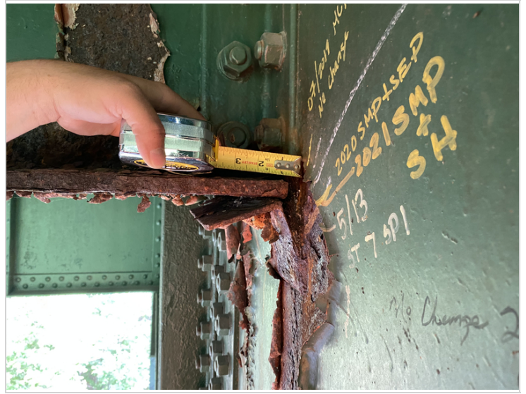
Cracked Weld at Floor Beam #1 West Side along Beam #7
