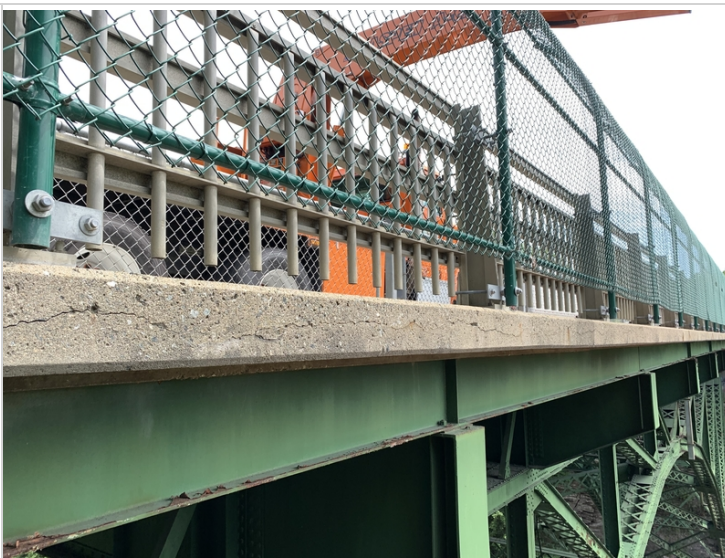
Cracking along Downstream Fascia
