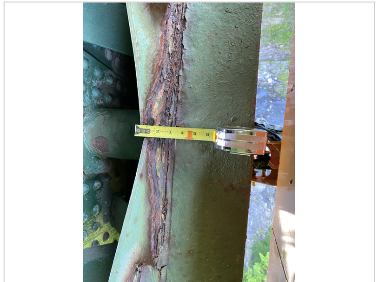
Pack Rust at Upstream Pin at Center of Arch
