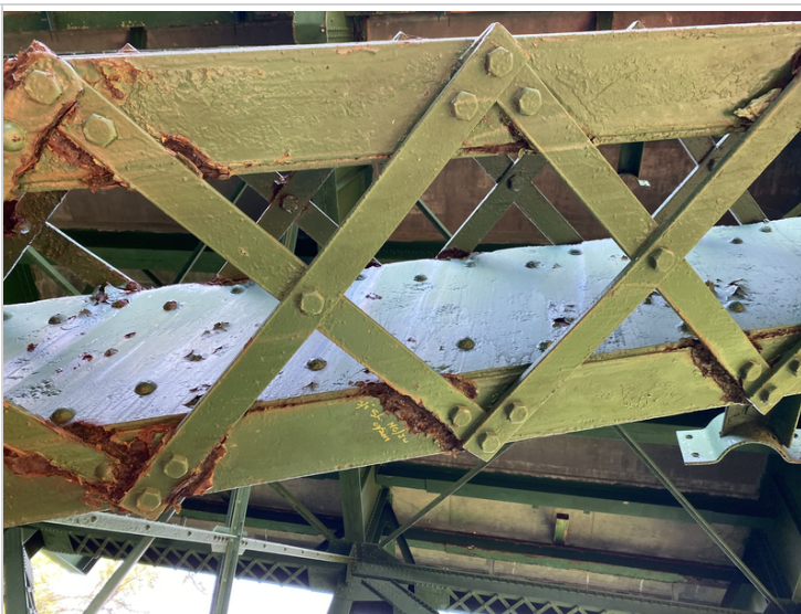
Bottom Chord #8 Pitting Upstream
