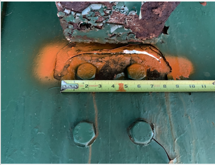
Crack/Perforation in Floor Beam Web #6 from East Side on Stringer #2
