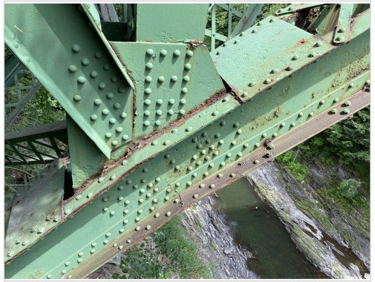
Bottom Chord Gussets along Downstream Side at Vertical #2
