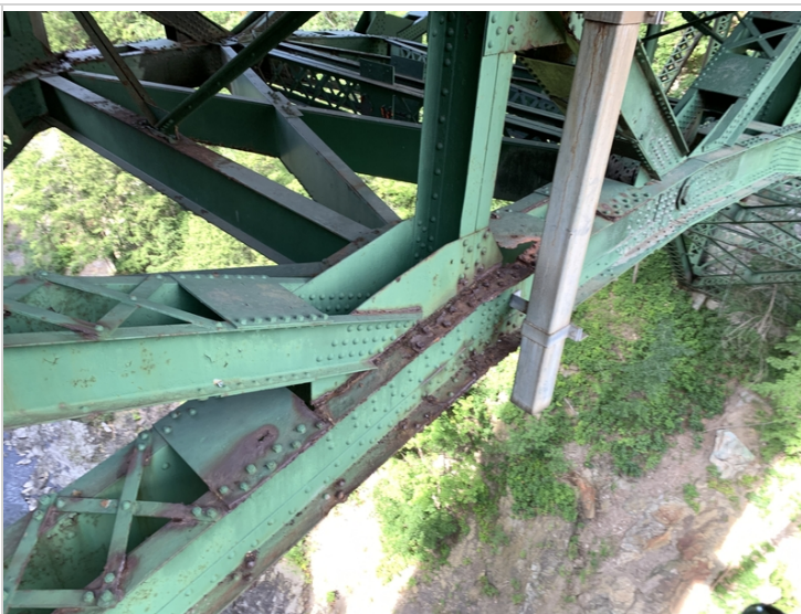
Bottom Chord at Vertical #6 Gusset / Connection Plate with Section Loss
