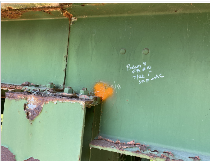
Beam #8 at Floor Beam #10 Downstream with ~1" Crack at Coped End
