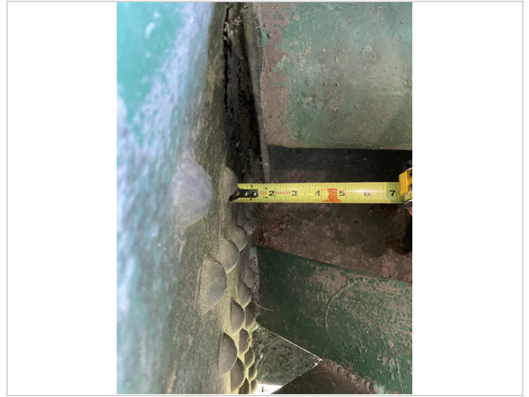
Upstream Center Pin Plate Deformation
