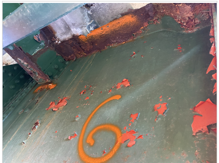
Floorbeam #6 Upstream Top Flange with Perforations East Side
