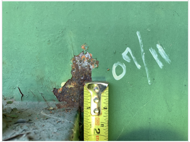
Crack in Stringer #8 at Floor Beam #10 ~1" in Height on Bottom of Coped End
