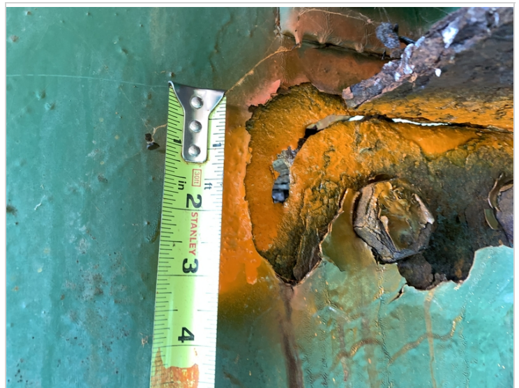
Crack along Web on Downstream side of Floorbeam #6 below Connection with Stringer #7
