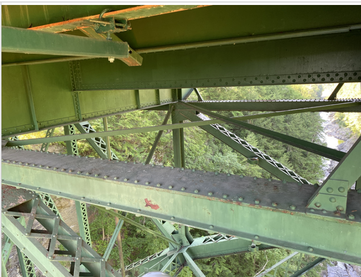
Top Chord Pitting between Floor Beams #7 and #8
