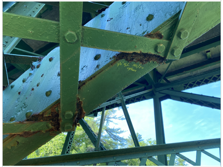
Bottom Chord Pitting between Verticals #8 and #9 Upstream
