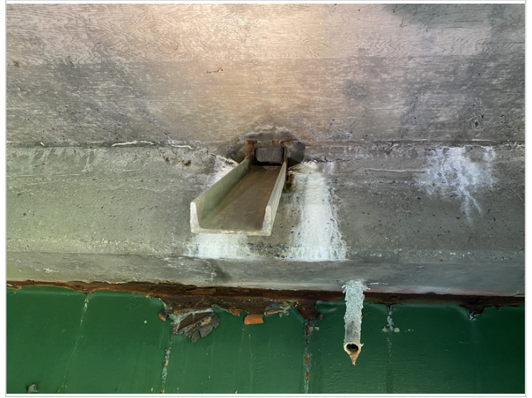
Typical Deck Scupper / Weep Tube / Efflorescence Leakage
