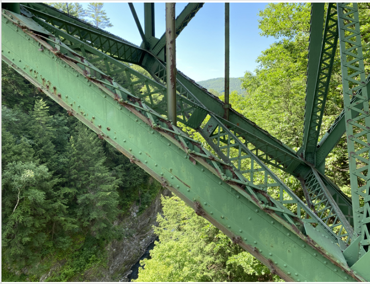
Bottom Chord between Vertical #2 and #3 Upstream
