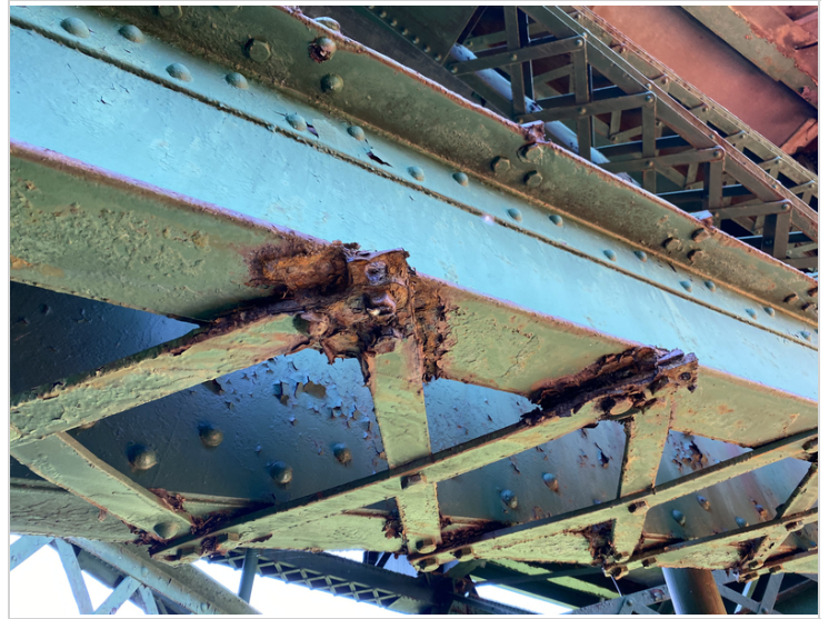
Bottom Chord Section #6 Upstream Pitting / Rust Scaling
