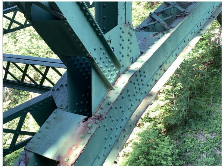
Section Loss in Plating at Vertical #9 Upstream on Bottom Chord
