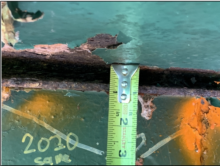
~3/4" Movement of Connection Plate on Stringer
