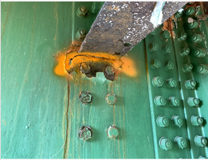
Crack along Web on Downstream side of Floorbeam #6 below Connection with Stringer #7 on East Side
