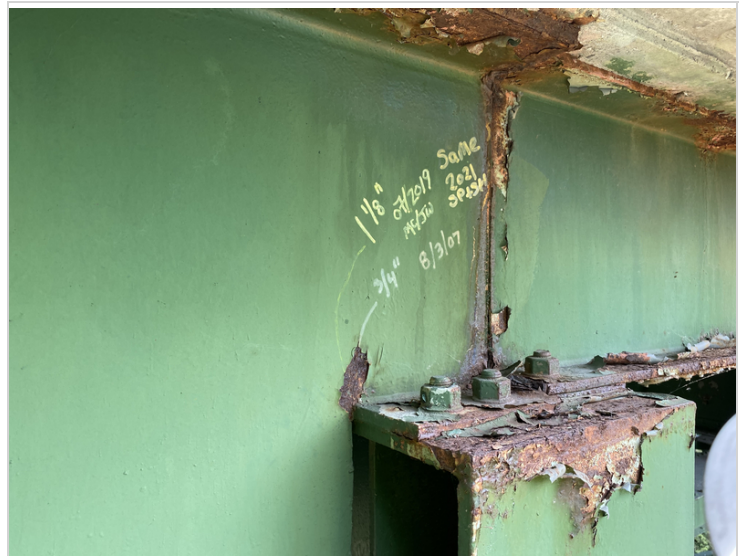
Girder #8 over Floor Beam #1 with ~1-1/8" Crack
