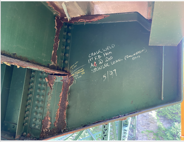
Cracked Weld at Floor Beam #1 West Side along Beam #7
