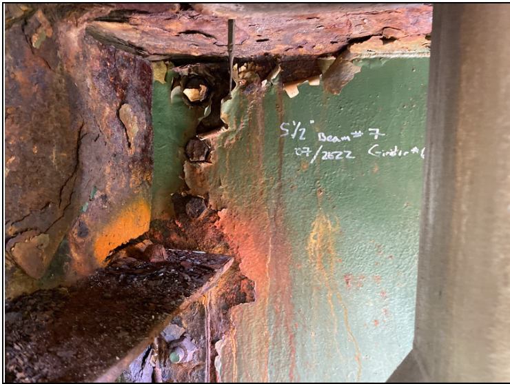
~5-1/2" Perforation along Lower Portion of Web on
