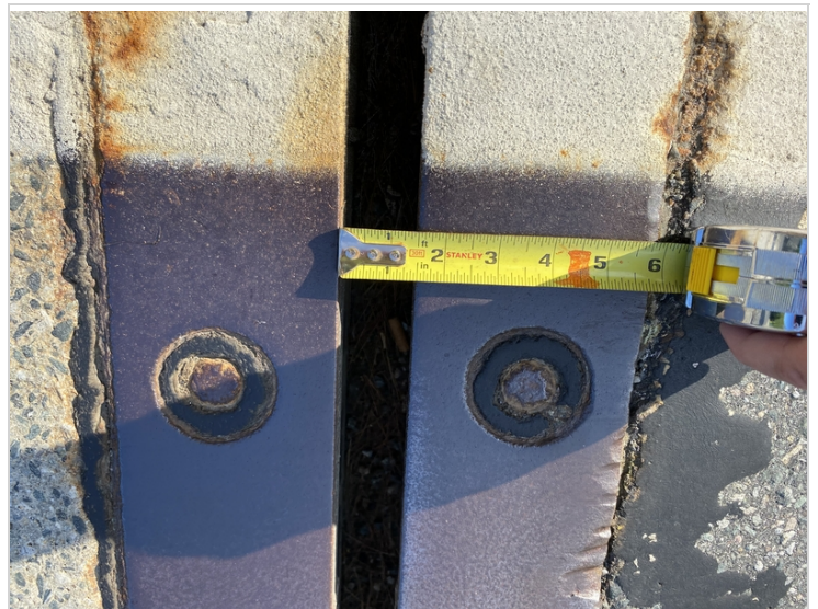
Vermont Type Joint over Abutment #2 Separation
