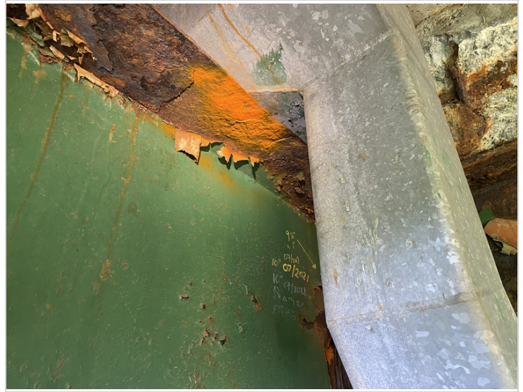
Floorbeam #6 Upstream Top Flange with Perforations West Side
