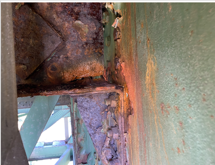
~5-1/2" Perforation along Lower Portion of Web on Beam #7 at Floor Beam #6
