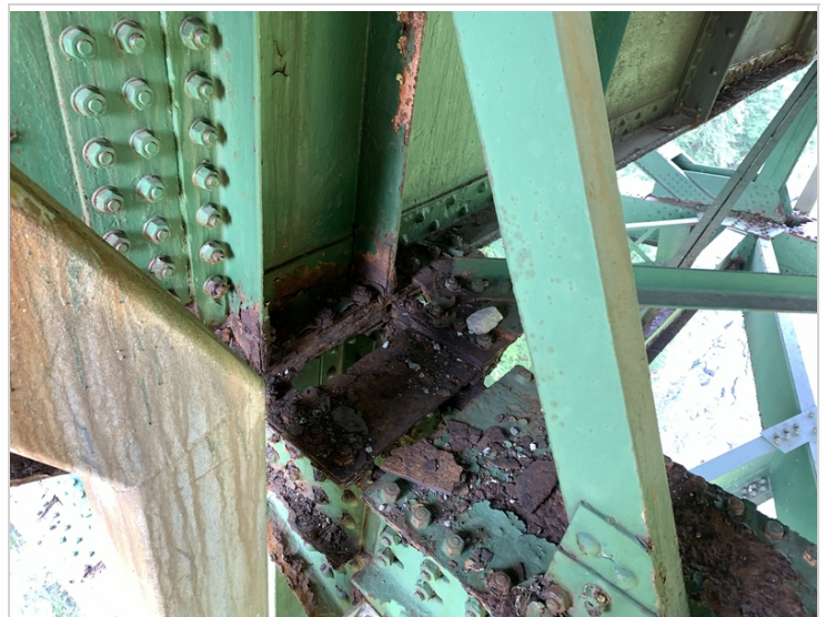
Rust Scaling on Top Chord below Floor Beam #6 on West Side
