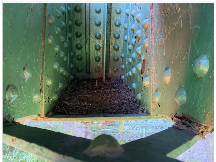
Heavy Debris Build Up at Vertical #8 Upstream
