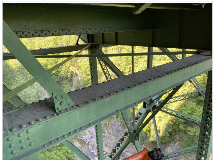
Top Chord Pitting between Verticals #9 and #8 Upstream
