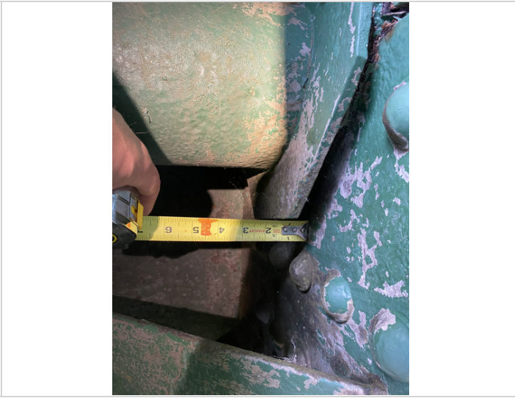
Upstream Interior Plate Bending / Displacement at Center Pin
