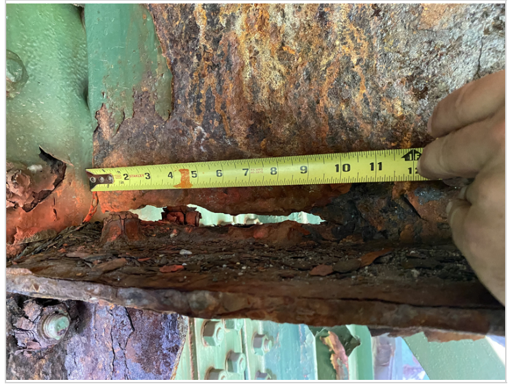
~10" Perforation along Lower Portion of Web at Beam #2 at Floor Beam #6
