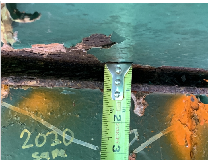
~3/4" Movement of Connection Plate on Stringer #7 at Floor Beam #10
