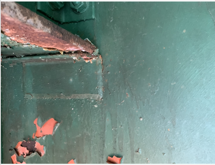
Cracking in Weld at Floor Beam #10
