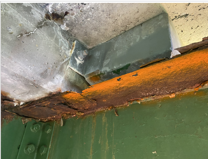
Floorbeam #6 Upstream Top Flange with Perforations East Side
