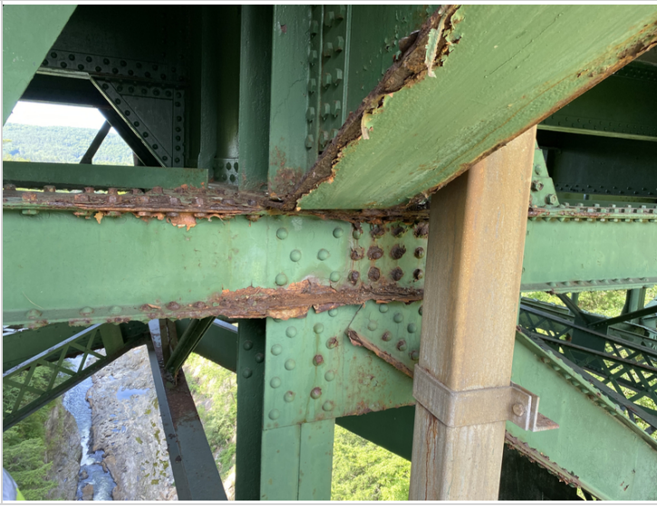
Upstream Top Chord at Floor Beam #6 / Gusset
