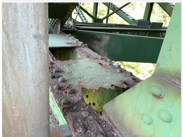
Section Loss along Upstream Bottom Chord Connection Plate between Vertical #4 and #5
