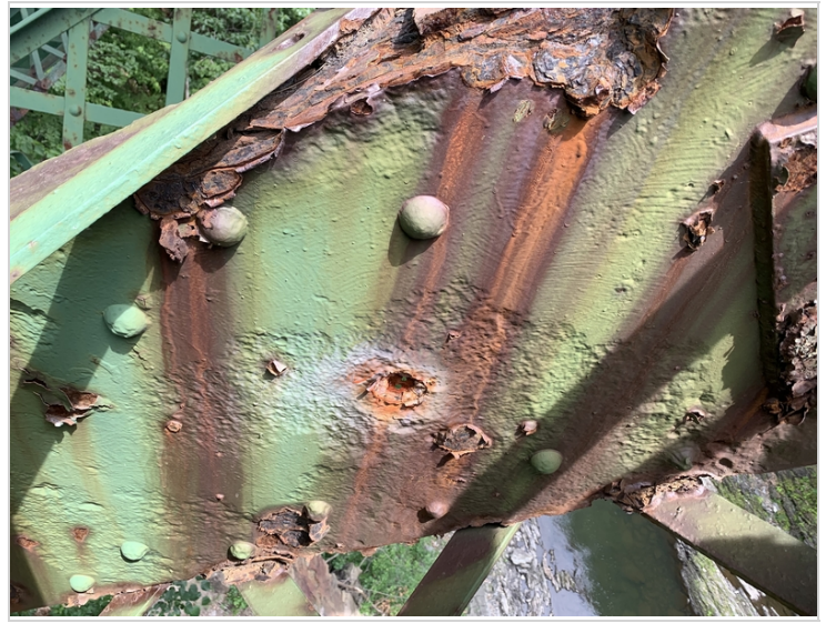
Downstream Bottom Chord with Section Loss and Pitting between Verticals #2 and #3
