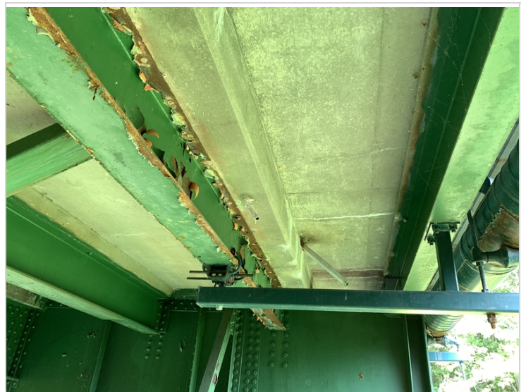
Cracking in Deck Underside
