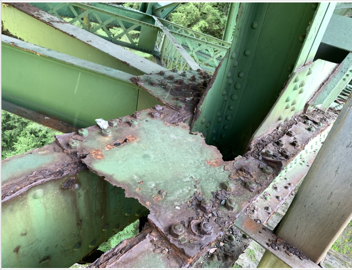
Section Loss along Upstream Bottom Chord Connection Plate between Vertical #4 and #5
