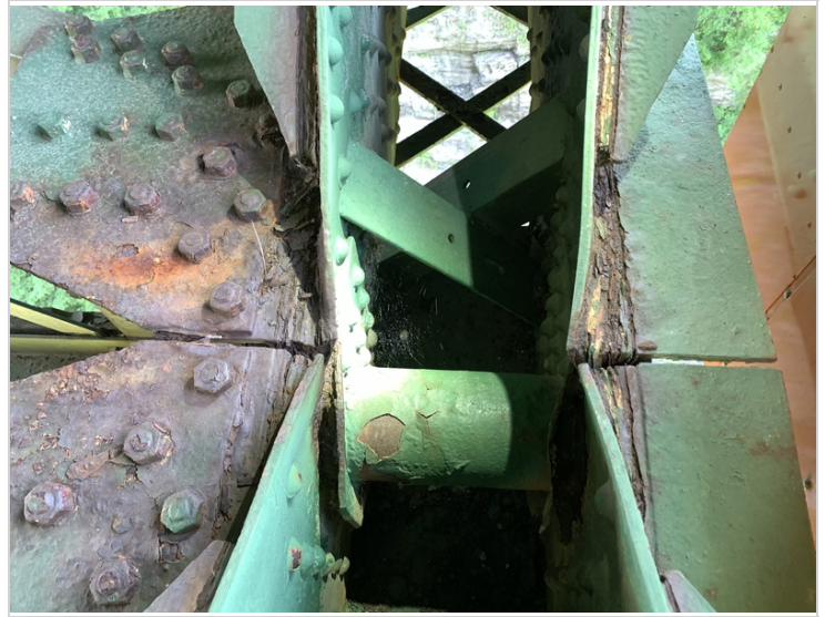
Downstream Pin Condition
