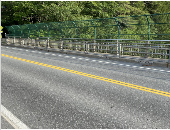
Upstream Curb Spalling
