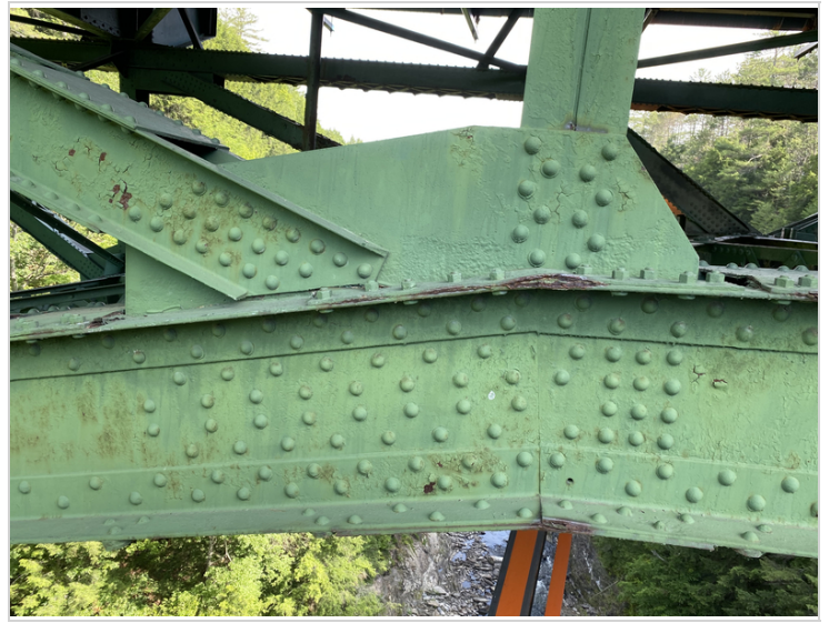
Downstream Bottom Chord / Gusset at Vertical #5
