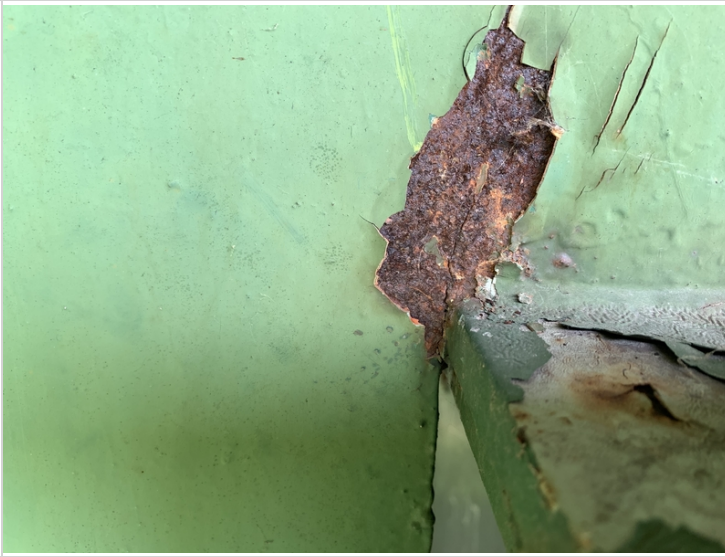
Crack in Stringer #8 at Floor Beam #1 ~1-1/8" in Length
