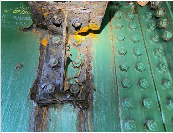
Lower Connection at Floor Beam #6 on Beam #2 West Side
