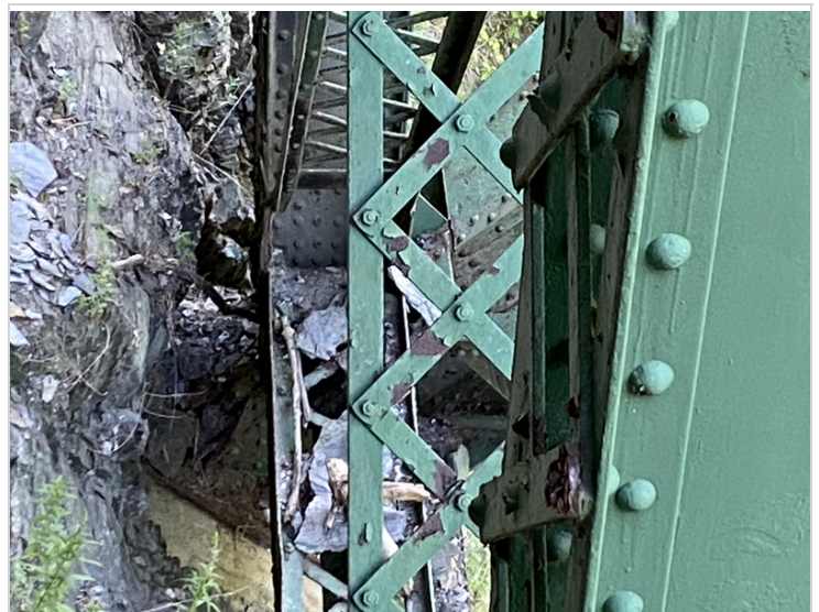
Build Up of Debris on Downstream Bearing / Cross Bracing below Vertical #10
