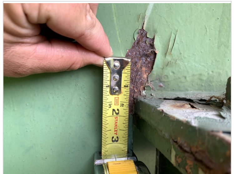
Crack in Stringer #8 at Floor Beam #1 ~1-1/8" in Length
