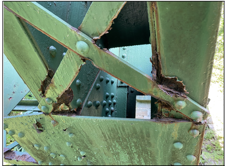
Bottom Chord Section Loss at Vertical #2 Upstream
