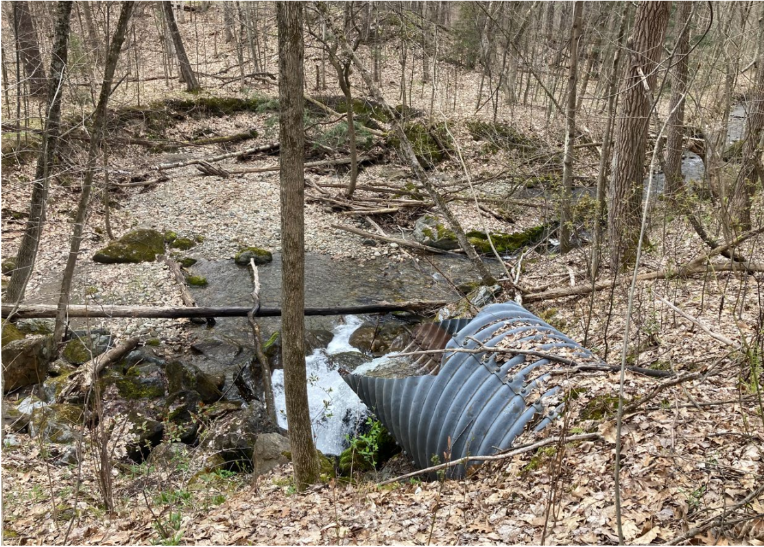
View of outlet end and scour area from slope. Portions of the lower level terrace can be seen beyond the scour area before the land rises to the higher terrace.
