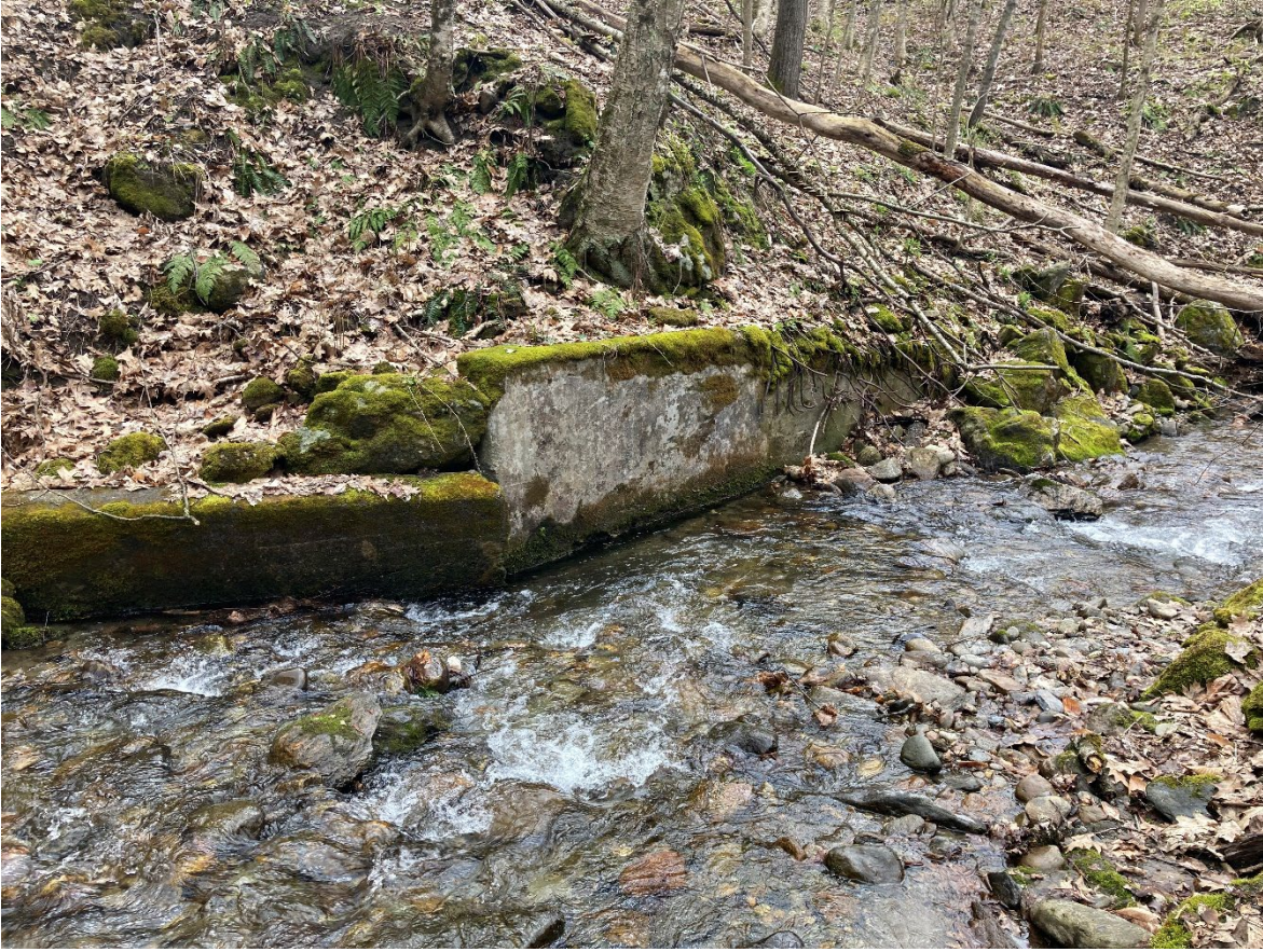
Concrete “wingwall” on east bank upstream of inlet (view from west bank upstream of inlet).
