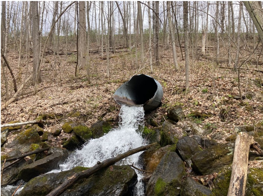
View of outlet end from base of slope looking upward toward I-89
