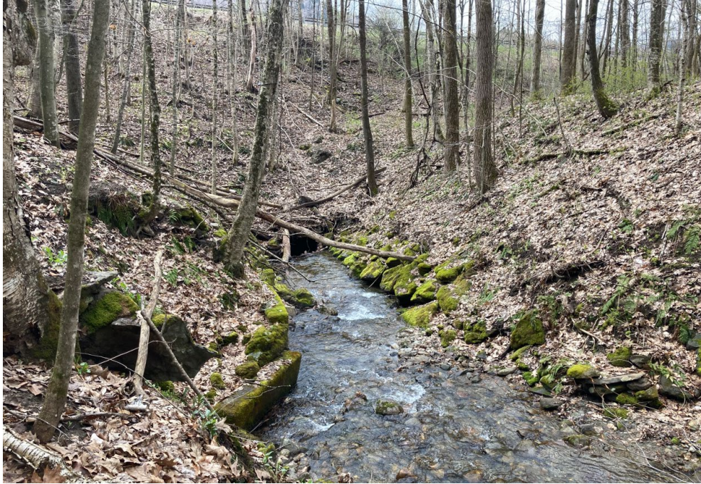
Image of culvert at north (inlet) end. Note concrete slabs center left and row of stones (rip rap) center right of stream channel
