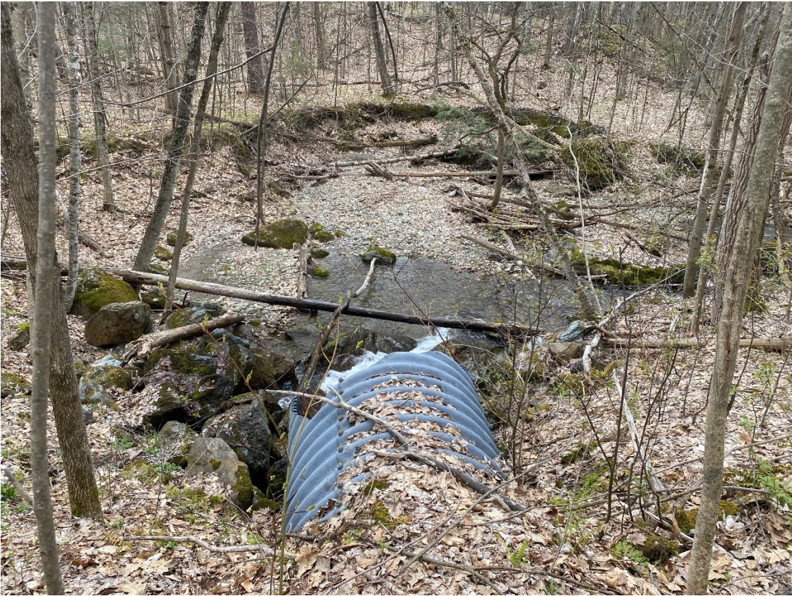
Looking southwest over the outlet at scour hole.
