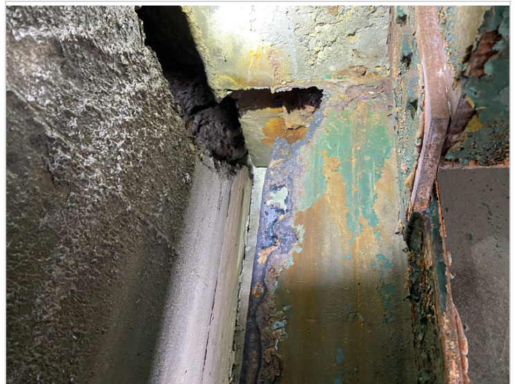
Girder #1 Perforation Behind Bearing Area at Abutment #1
