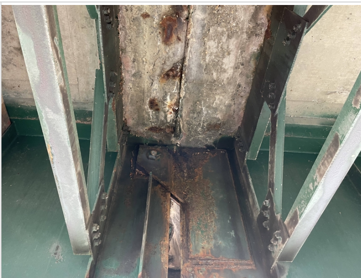
Underside of Concrete at Joint over Second Pin in Span #2
