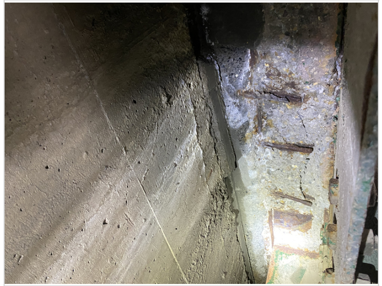
Spalling along Backwall / Deck Soffit over Abutment #1
