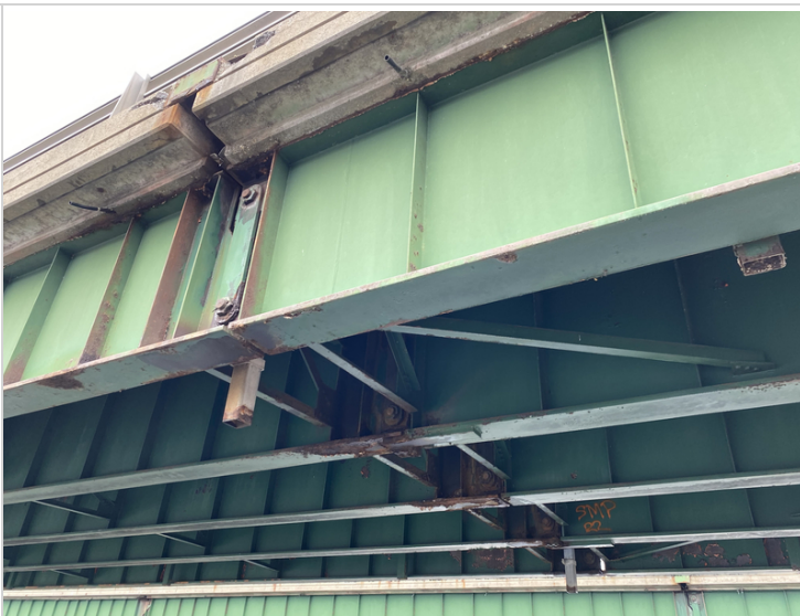
Girder #1 Span #2 First Pin Section / Deck Spalling
