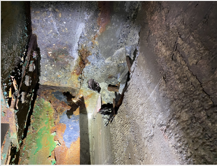
Girder #5 Corrosion at Abutment #1
