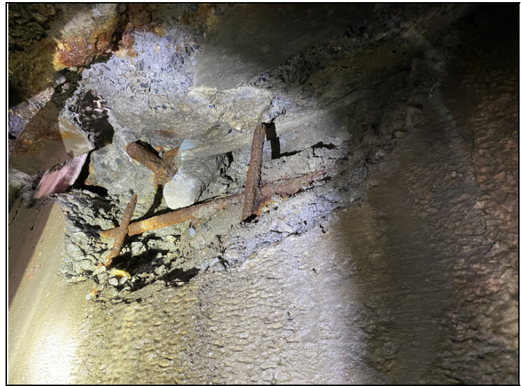
Backwall Spalling Abutment #1 East End Behind Girder #5
