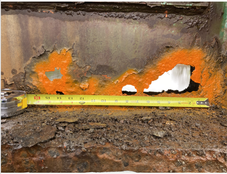
Beam #5 Perforations and section loss present at second section of Pins in Span #2
