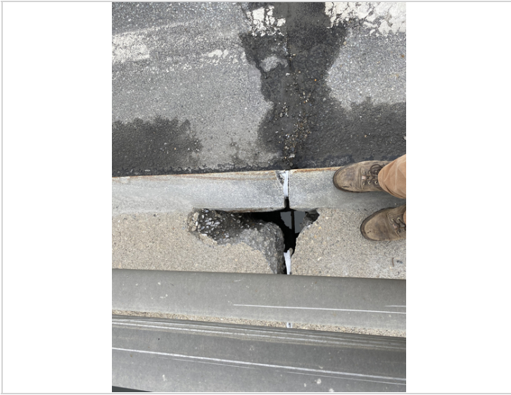
Full Depth Hole over Abutment #2
