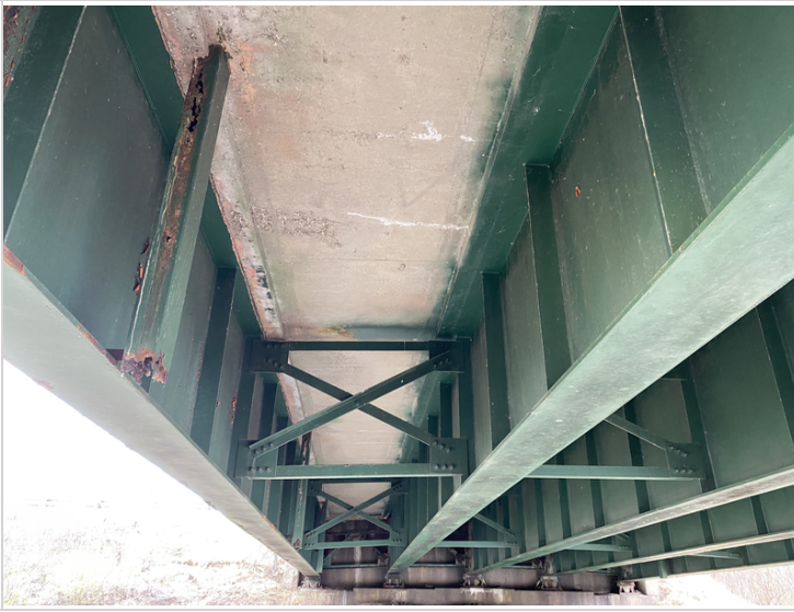
Bay #4 Deck Soffit / Deck Drains with Severe Corrosion
