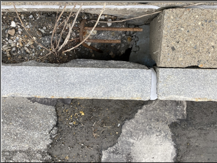
Spalling along Eastern Curbing over Abutment #2
