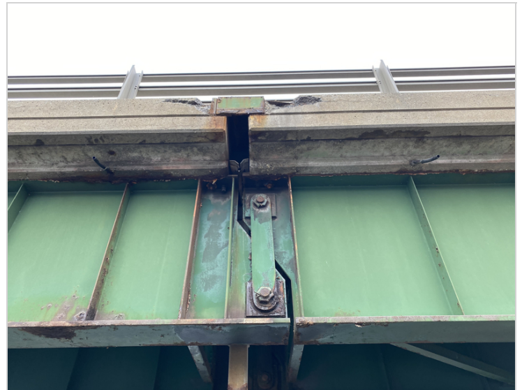
Girder #1 Span #2 First Pin Section / Deck Spalling
