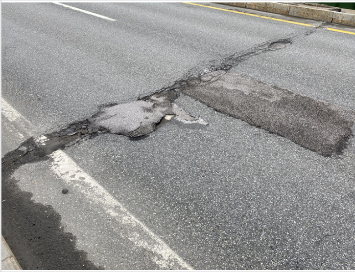
Joint / Asphalt over Second Pin Section in Span #2
