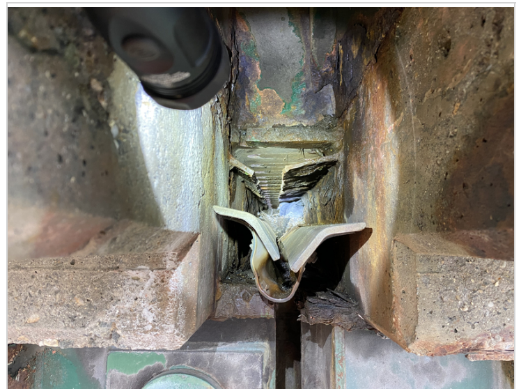
Heavy Debris in Trough at First Pin Section in Span #2
