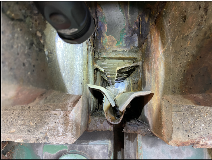
Heavy Debris in Trough at First Pin Section in Span
