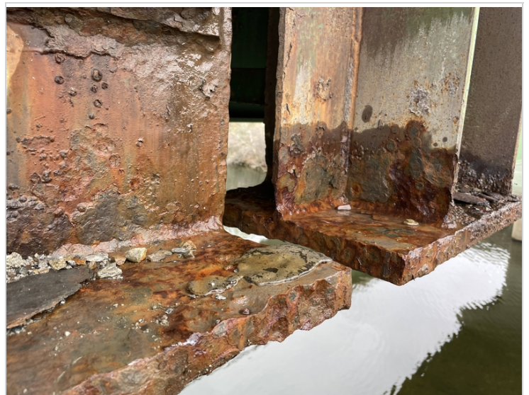
Pitting along Lower Flanges of Beam #1 in Span #2 at Northern Pin
