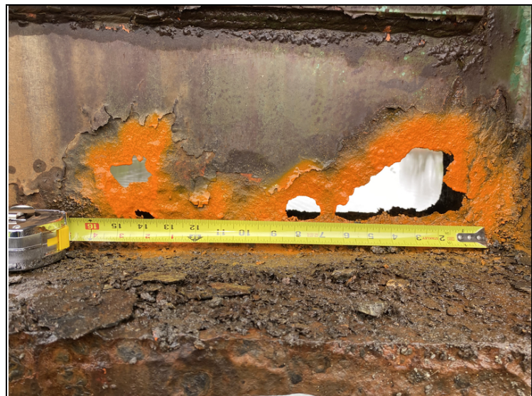
Beam #5 Perforations and Section Loss Present at Second Section of Pins in Span #2
