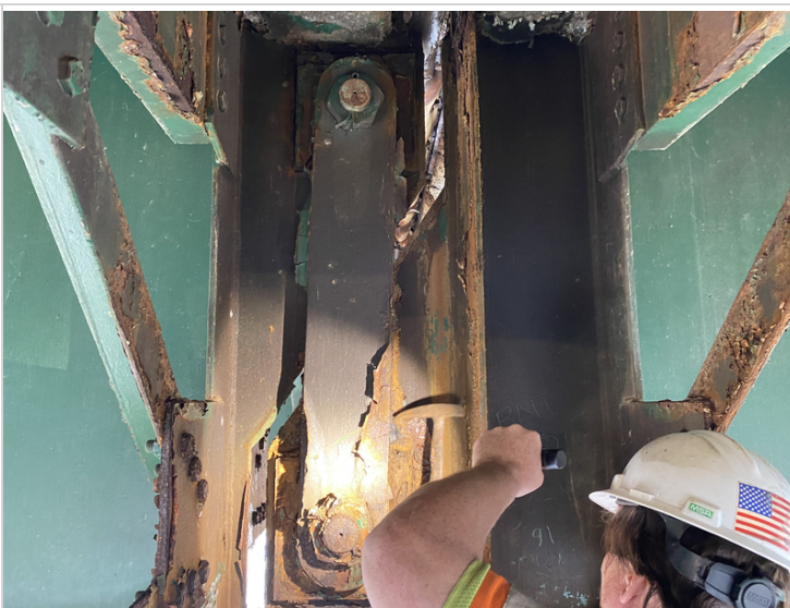
Girder #3 at First Section of Pins in Span #2 with Heavy Rust Packing and Scaling / Pitting
