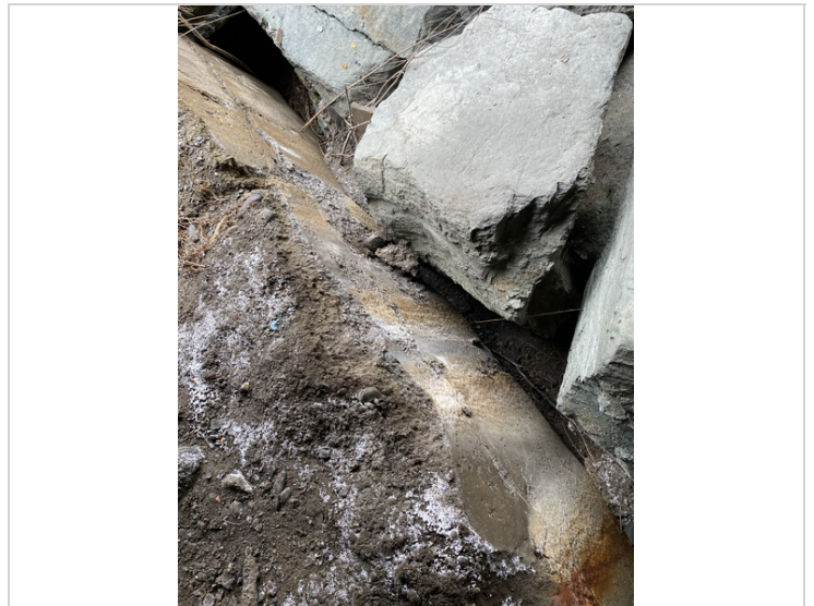
East End Abutment #2 Undermining
