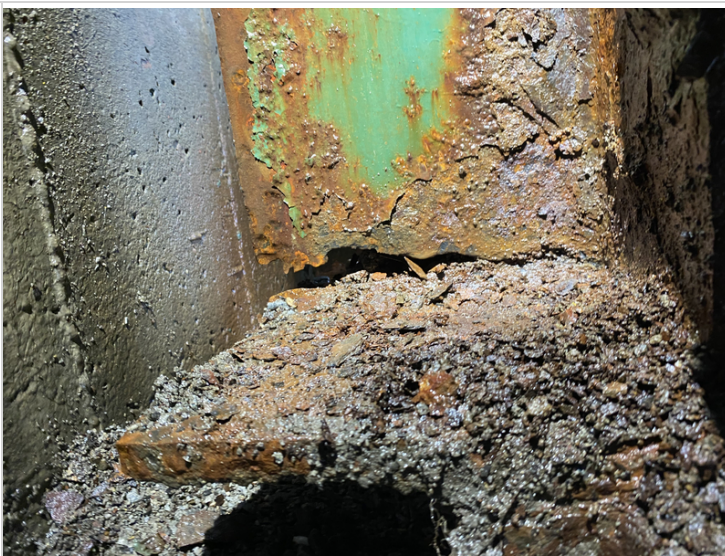
Girder #5 at Abutment #2 Perforation
