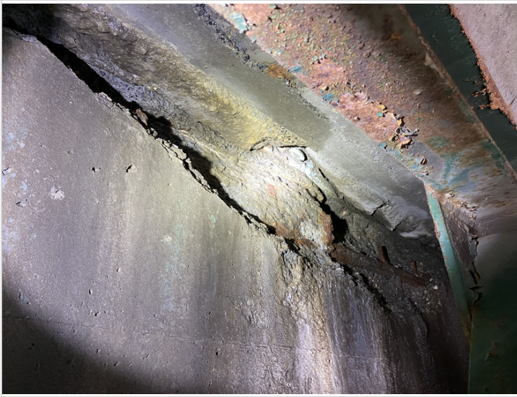
Spalling in Abutment #2 Backwall
