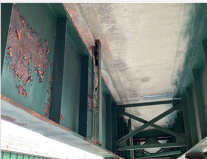
Severely Corroded Drain Downspout
