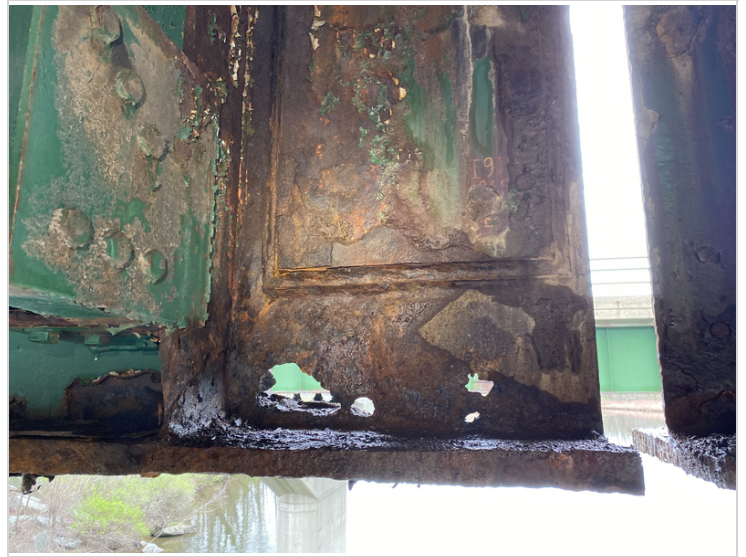
Beam #5 Perforations along Web in Span #2 Second Pin Section
