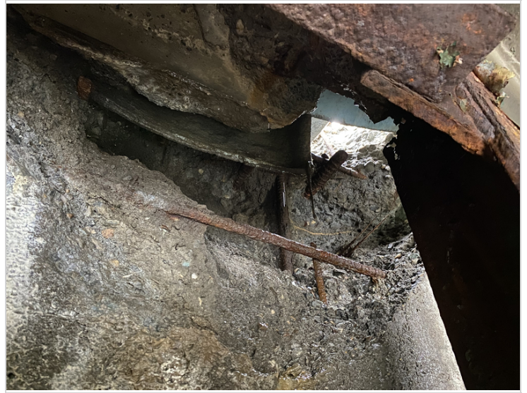
East End Abutment #2 Backwall
