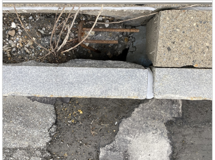
Spalling along Eastern Curbing over Abutment #2
