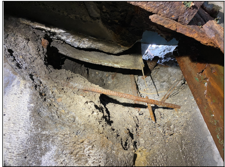
Backwall Spalling at Abutment #2 East End
