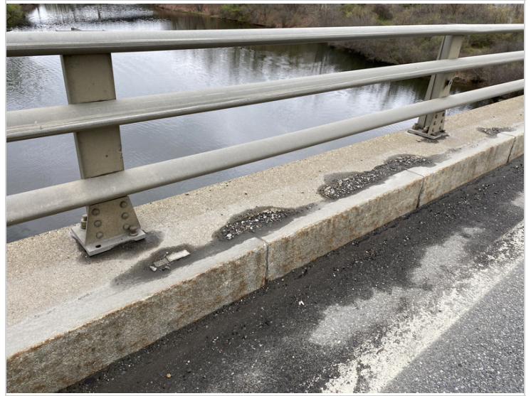
Damaged Anchor Bolts in Posts
