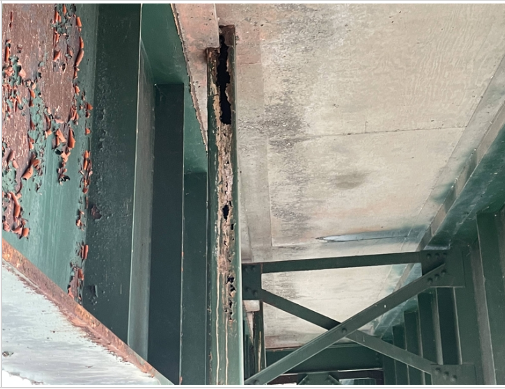
Rusted Through Drain
