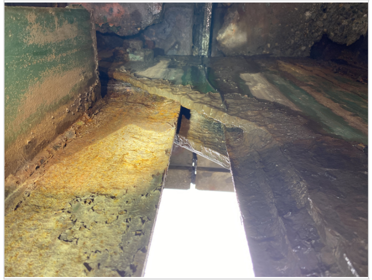
Severe Pitting / Measurable Section Loss Beam #1 at Second Pin Section Span #2
