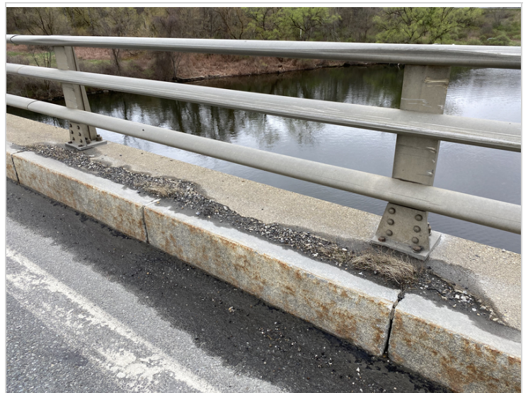
Aluminum Bridge Rail / Posts Scrapes / Gouges and Dents
