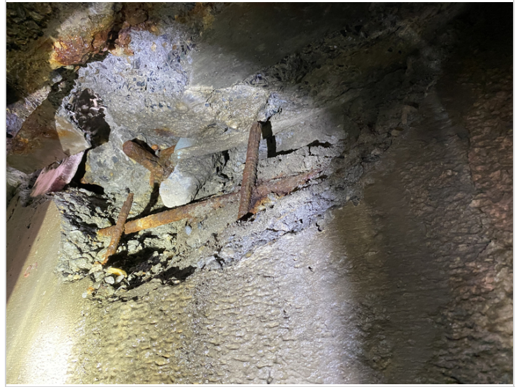
Backwall Spalling Abutment #1 East End Behind Girder #5
