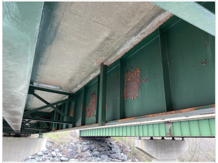
Girder #5 Protective System Peeling in Span #2
