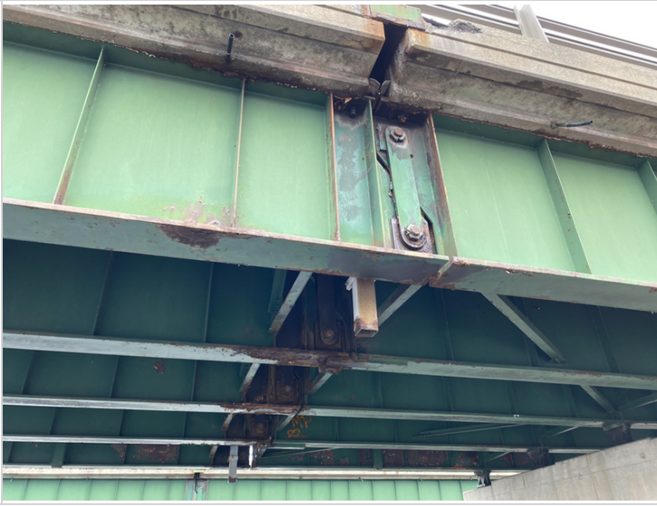
Girder #1 Span #2 First Pin Section / Deck Spalling
