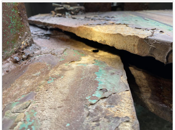
Small ~1" Perforation in Beam #5 at Second Section of Pins in Span #2
