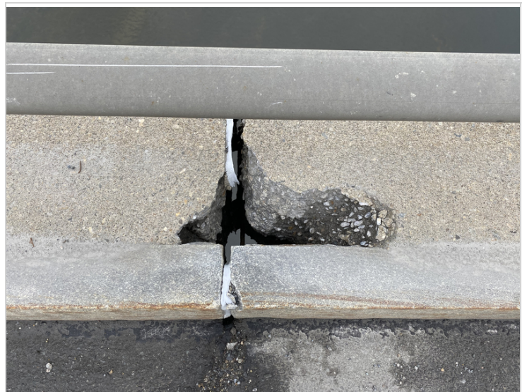
Full Depth Spalling along Curb
