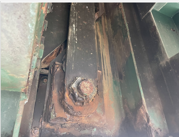
Beam #2 corrosion in Span #2 at First Pin Assembly
