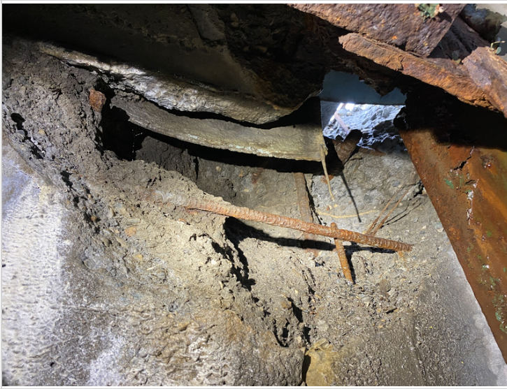
Backwall Spalling at Abutment #2 East End
