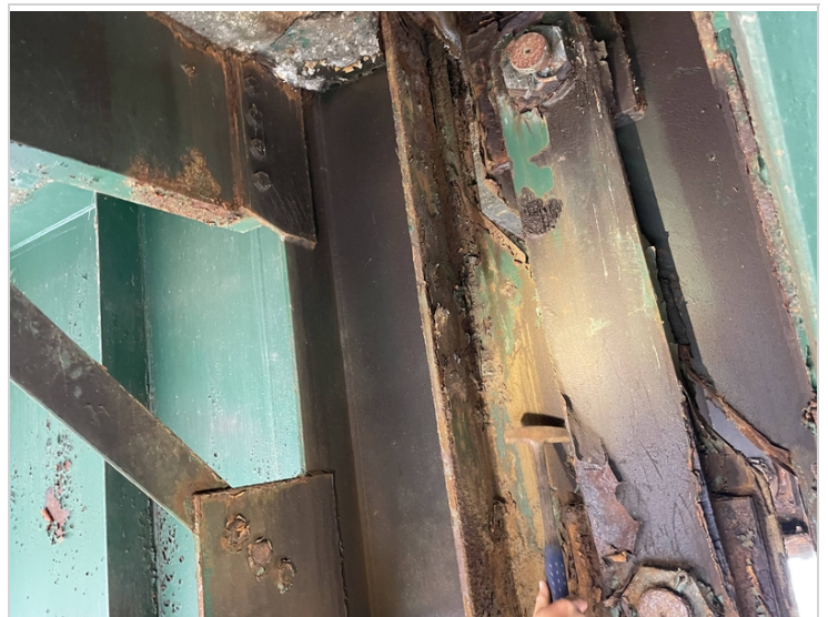
Beam #2 Pack Rust Behind Hanger Bars
