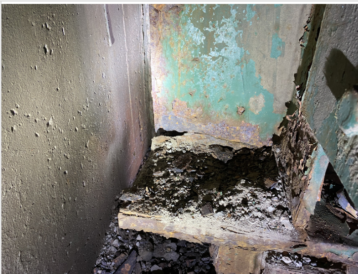
Girder #1 Perforation / Cracking Behind Bearing Area at Abutment #1
