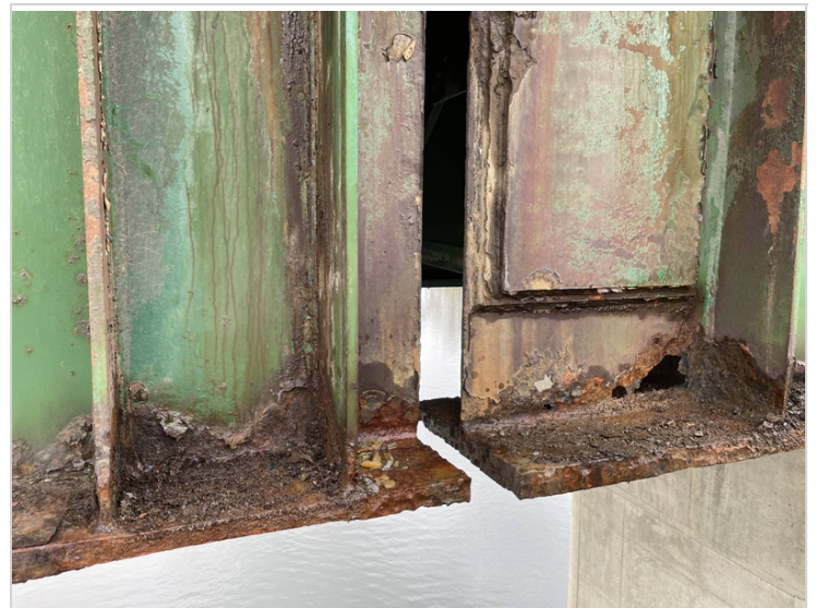
Beam #5 Section Loss in Span #2 at Second Set of Pins
