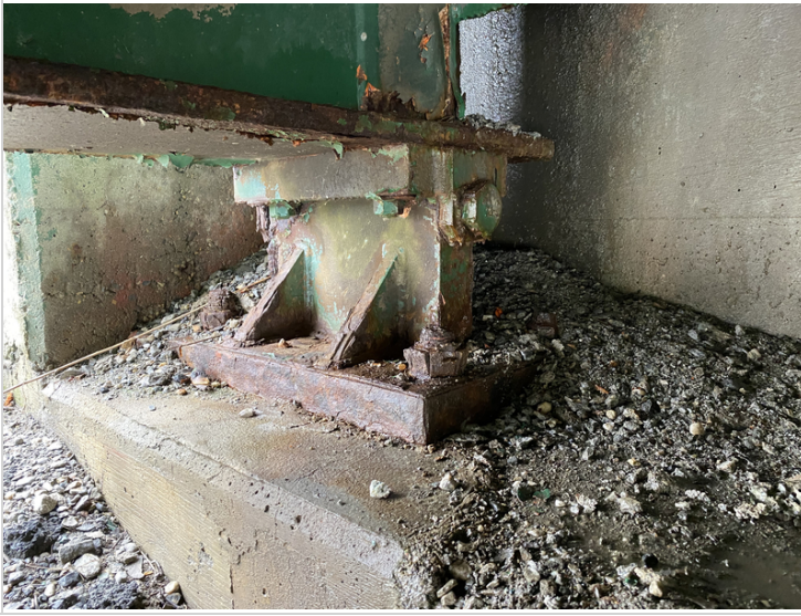
Bearing #5 at Abutment #1 with Heavy Debris Build Up
