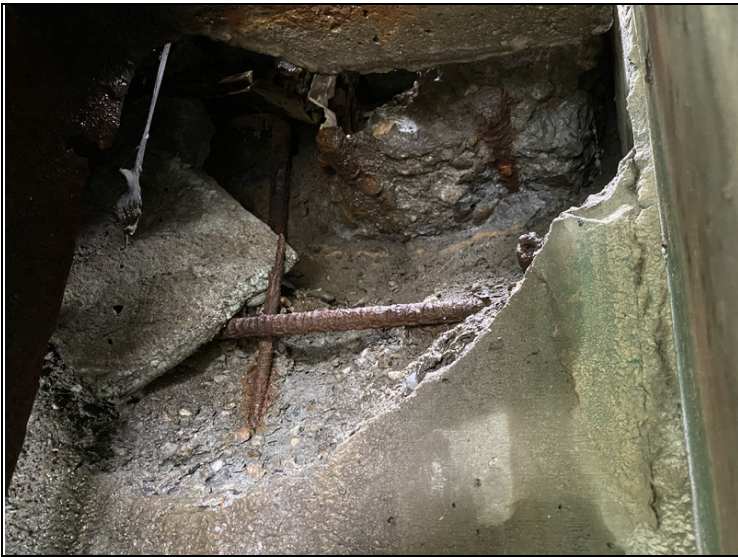
Spalling along Abutment #2 East Backwall
