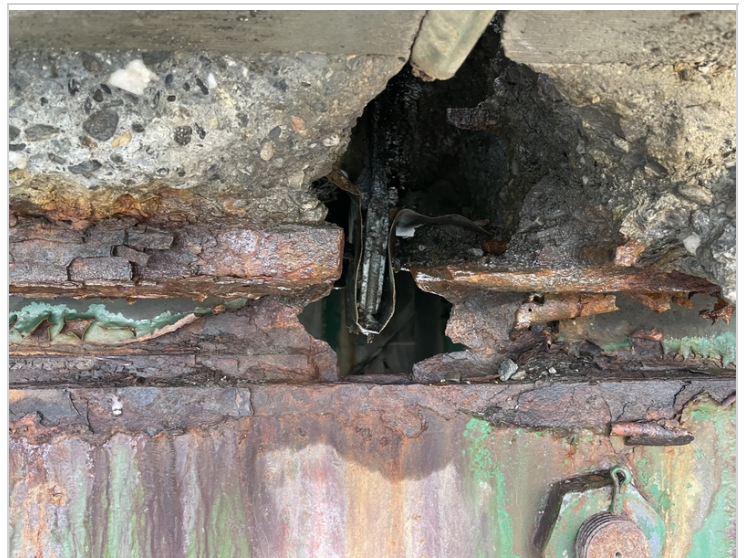
Pin Assembly Girder #1 Section Loss along Top Flange / Web and Deck Spalling
