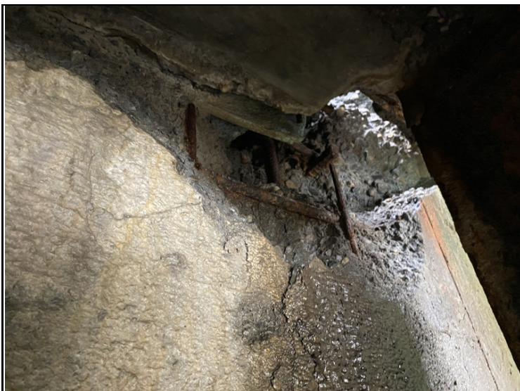
Heavy Spalling with Exposed Steel Reinforcing
