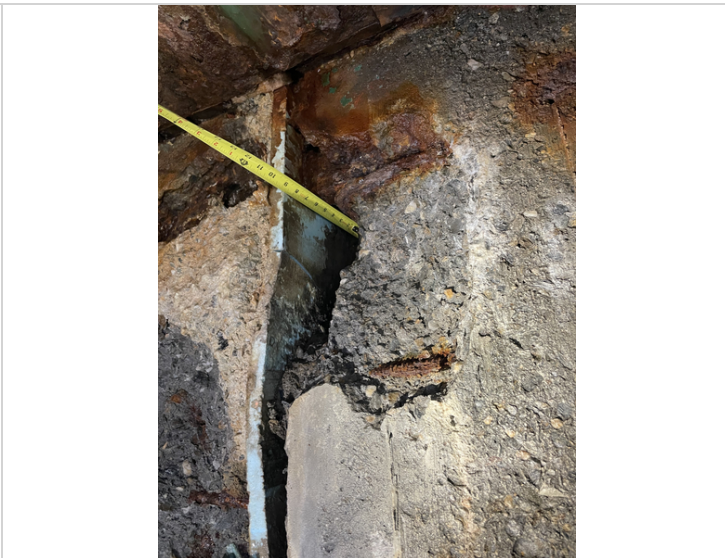
Deck Spalling over Second Section of Pins in Span #2
