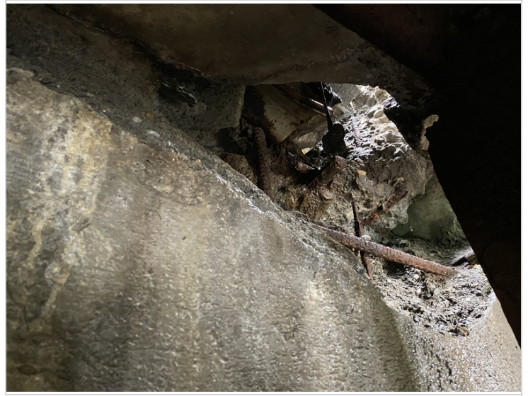
Spalling along Abutment #2 East Backwall
