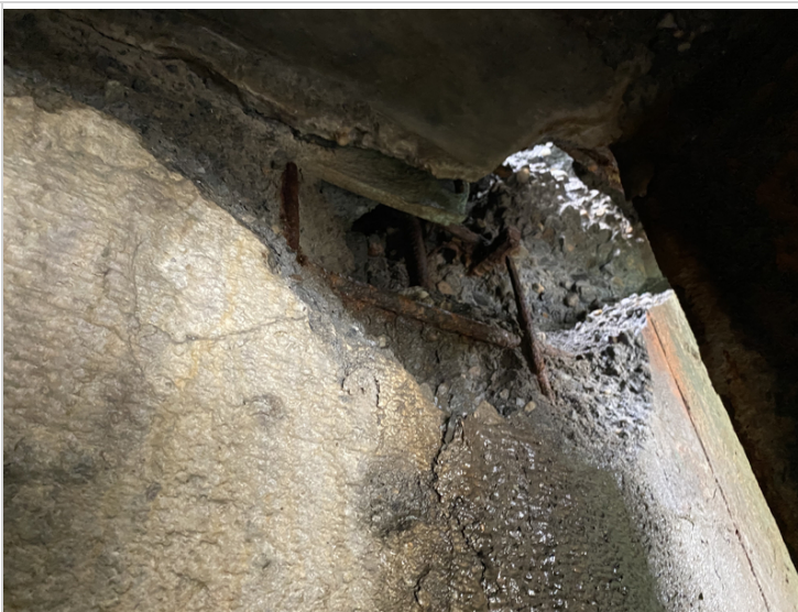
Heavy Spalling with Exposed Steel Reinforcing West End Abutment #1
