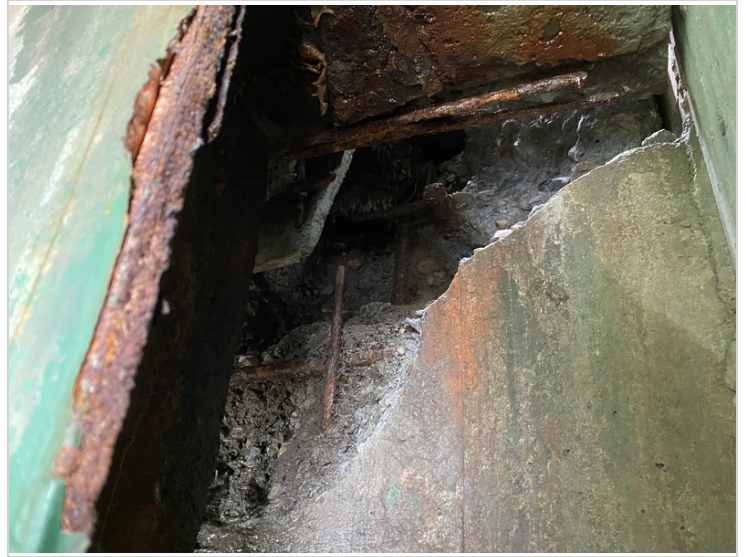
Heavy Spalling with Exposed Steel Reinforcing West End Abutment #1
