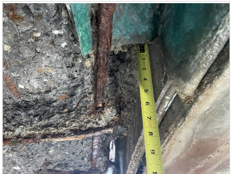
Spalling Depth at Second Section of Pins in Span #2
