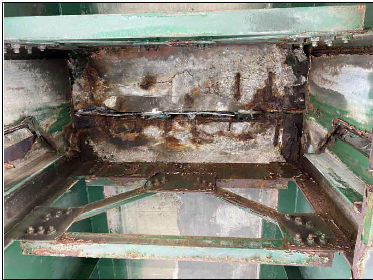
Deck Spalling over Second Section of Pins in Span
