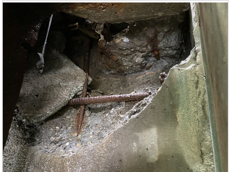
Spalling along Abutment #2 East Backwall
