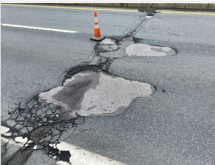
Heavy Break Up / Patches over Pin Section #2 in Span #2
