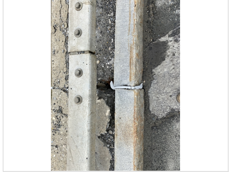
Curb Spalling along the East Side of Structure over Pier #1
