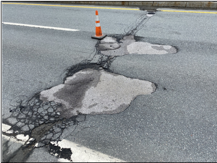
Heavy Break Up / Patches over Pin Section #2 in
