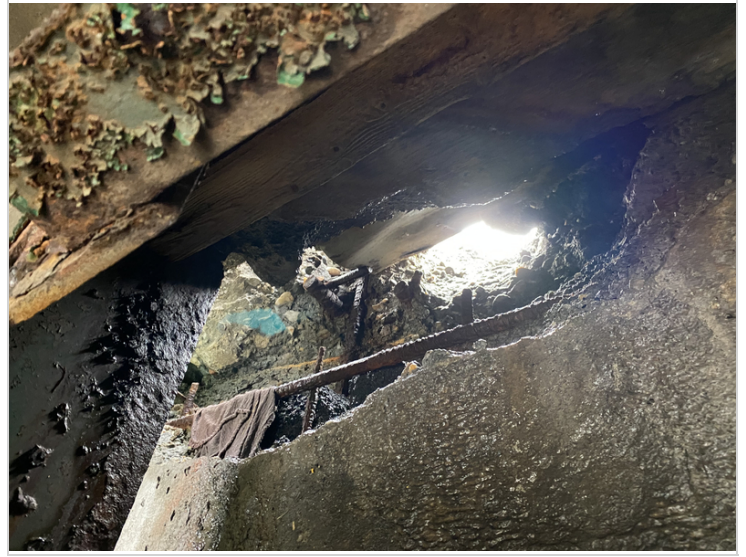
Full Depth Hole West Side of Abutment #2
