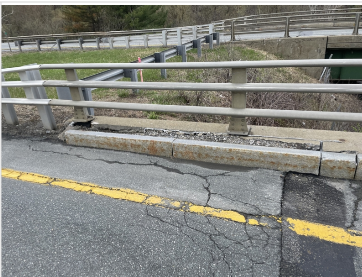
Spalling Curb along Southwest Corner
