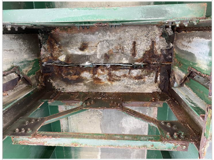
Deck Spalling over Second Section of Pins in Span #2
