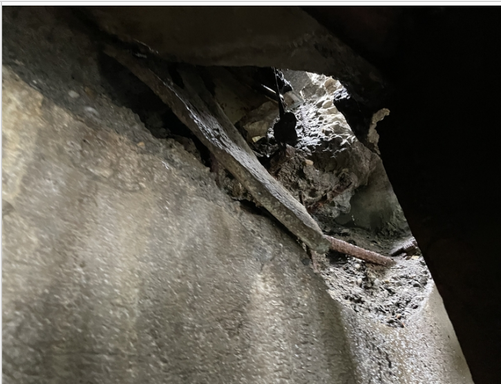
Hole Through Abutment #2 Backwall East Side
