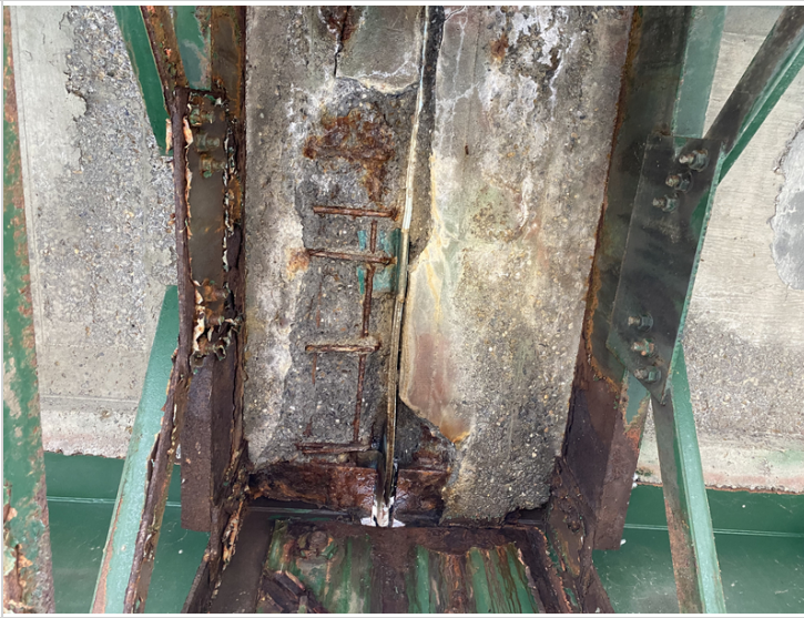
Deck Spalling over Second Section of Pins in Span #2 in Bay #1
