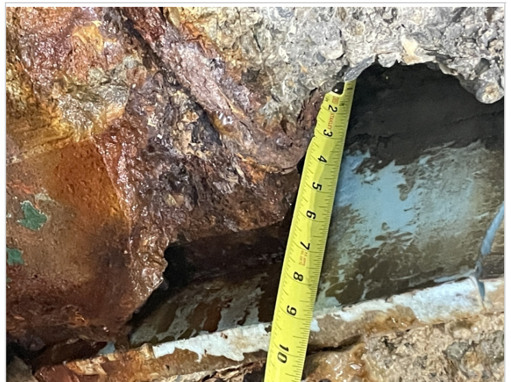
Deck Spalling at Second Section of Pins in Span #2
