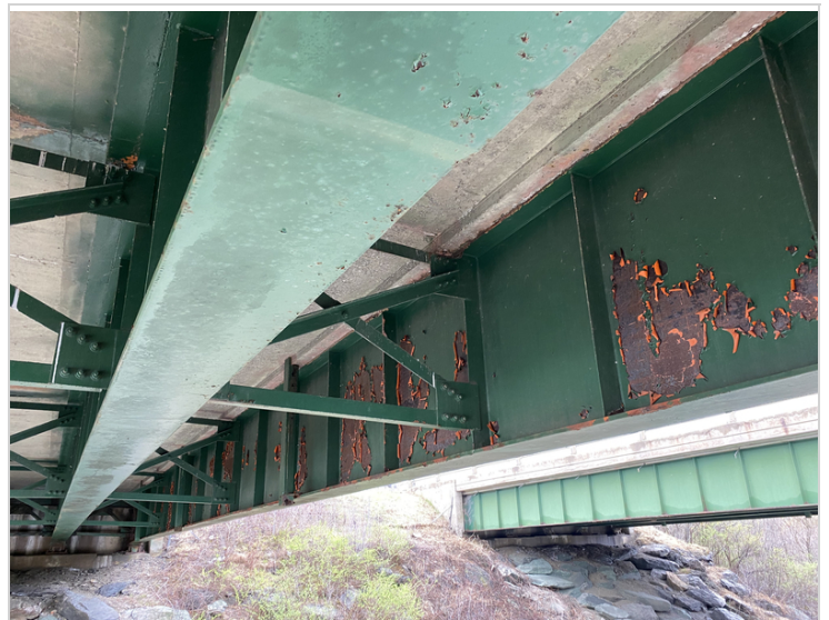
Girder #1 Span #1 Paint Peel
