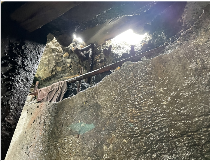
Hole Through Abutment #2 Backwall West Side
