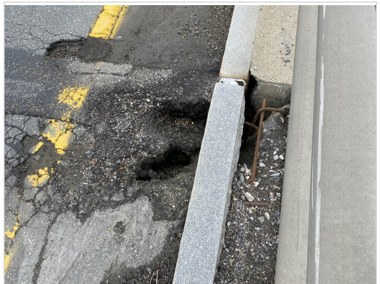
Full Depth Hole over West Shoulder at Abutment #2
