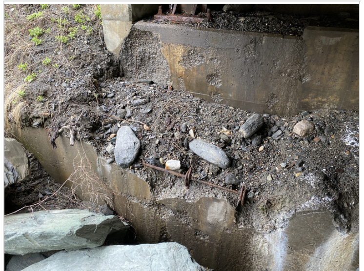
Heavy Spalling along Abutment #2 Footing
