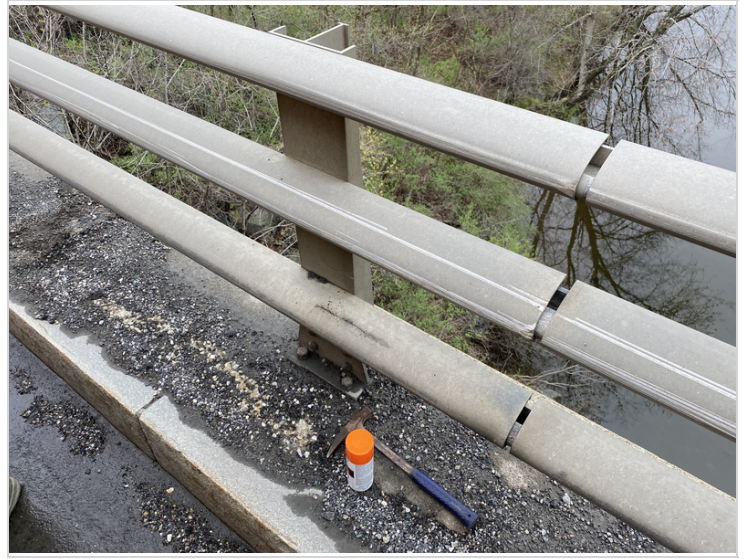
Typical Bridge Rail Scrapes
