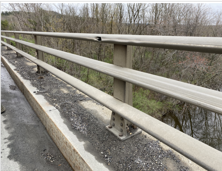
Typical Bridge Rail Scrapes
