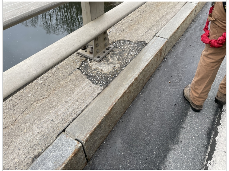
Patched Curb and Loose Anchor Bolts
