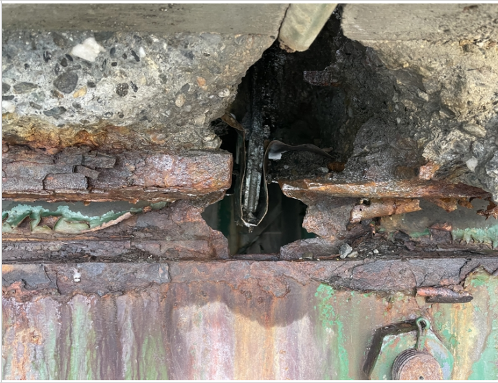
Pin Assembly Girder #1 Section Loss along Top Flange / Web and Deck Spalling
