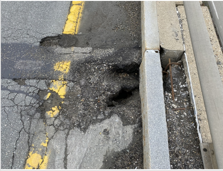
Full Depth Hole over West Shoulder at Abutment #2
