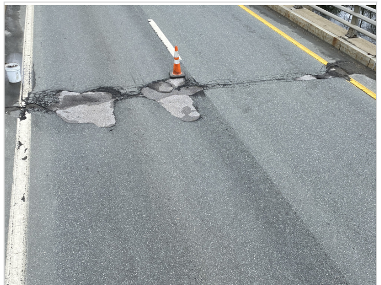
Breakup in Asphalt over Second Section of Pins in Span #2
