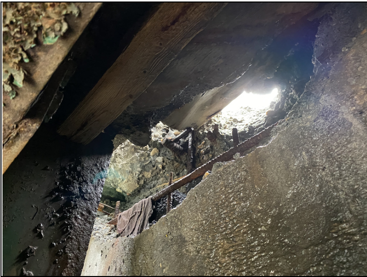
Full Depth Hole West Side of Abutment #2 ion
