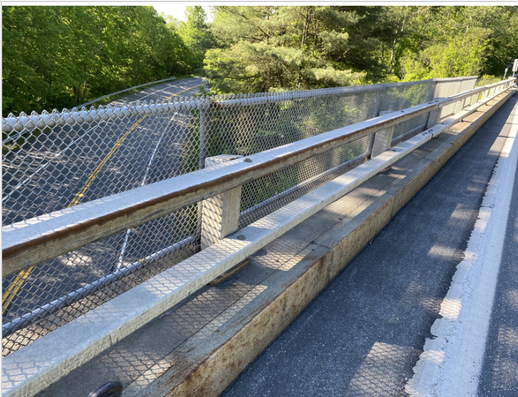
Bridge Rail Scraping / Dents on Eastern Side
