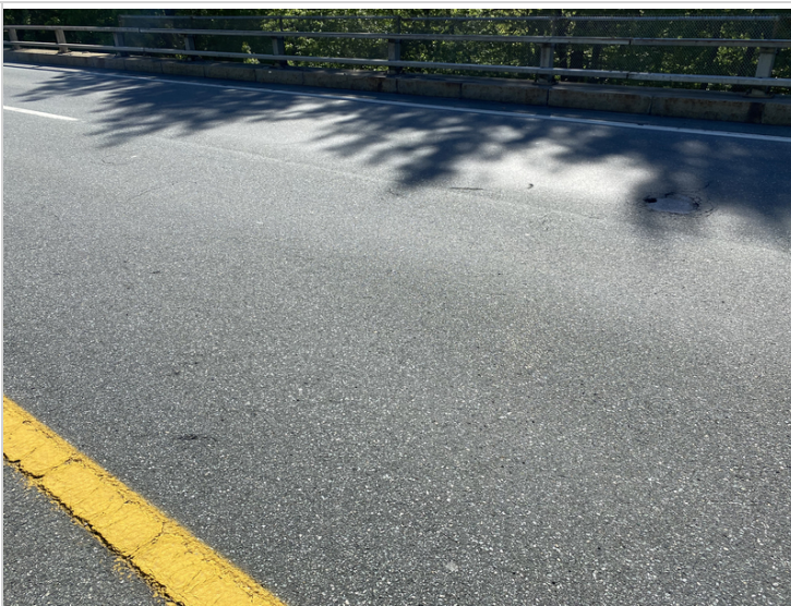
Pothole in Main Travel Lane with other Depression Nearby near South End of Span #2
