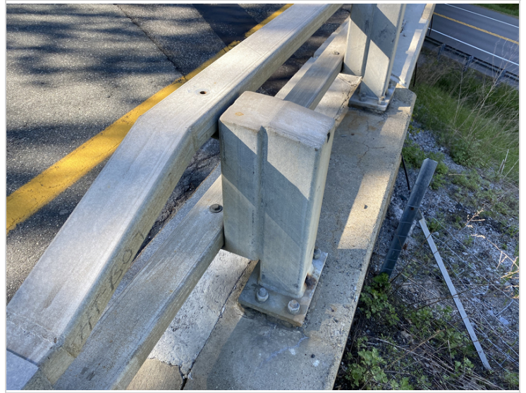
Missing Connection Bolt on Top Tier of Rail at Post #1 away from Abutment #2 on West Side
