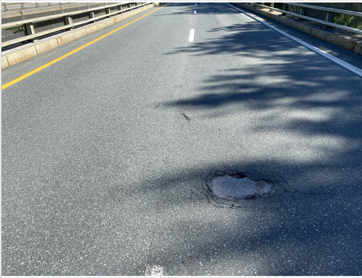
Pothole in Main Travel Lane with other Depression Nearby near South End of Span #2
