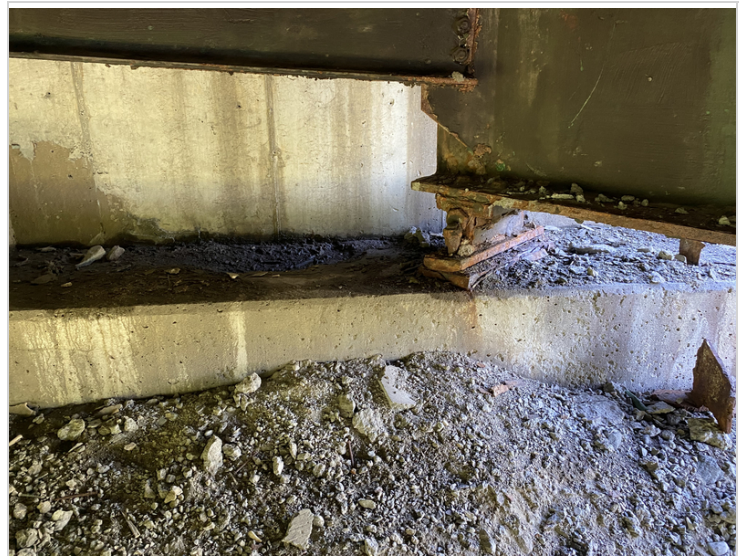
Abutment #1 West End / Bearing #1 / Bridge Seat Spalling
