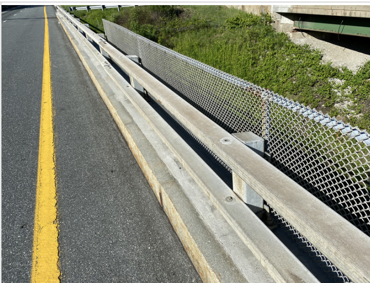
Missing Connection Bolts on Top Tier of Rail at Post #12 and #13 away from Abutment #1 on West Side
