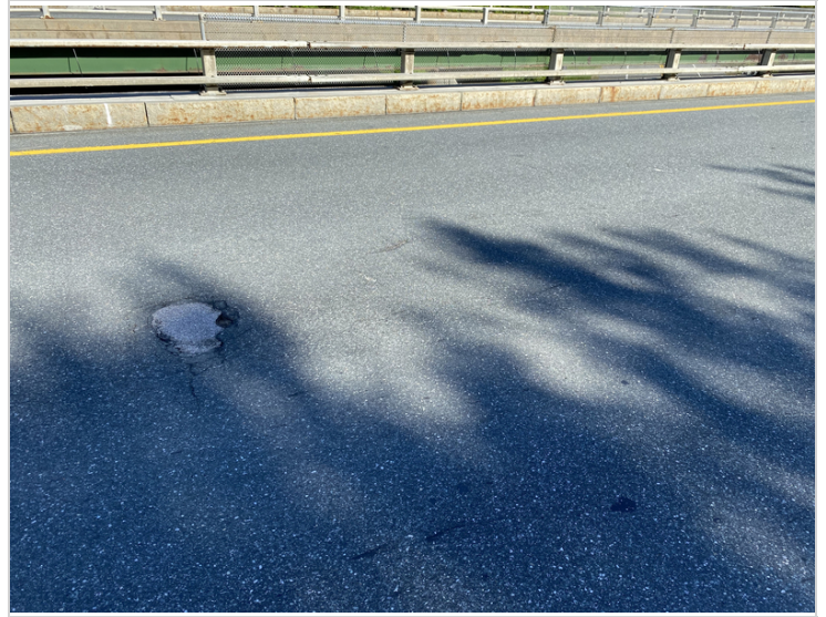
Pothole in Main Travel Lane with other Depression Nearby near South End of Span #2
