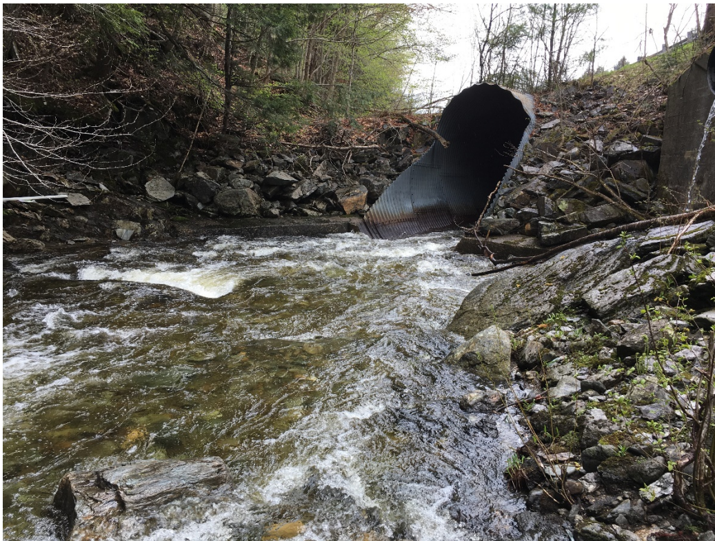
Figure 3.1: Exposed bedrock in the area of the inlet. [Structures photo dated April 2019]
