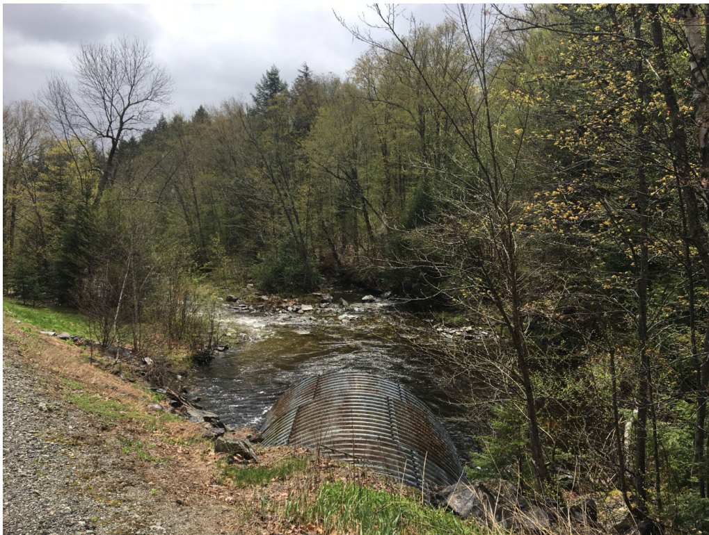
Picture 5: Looking Downstream (Note Scour Pool)
